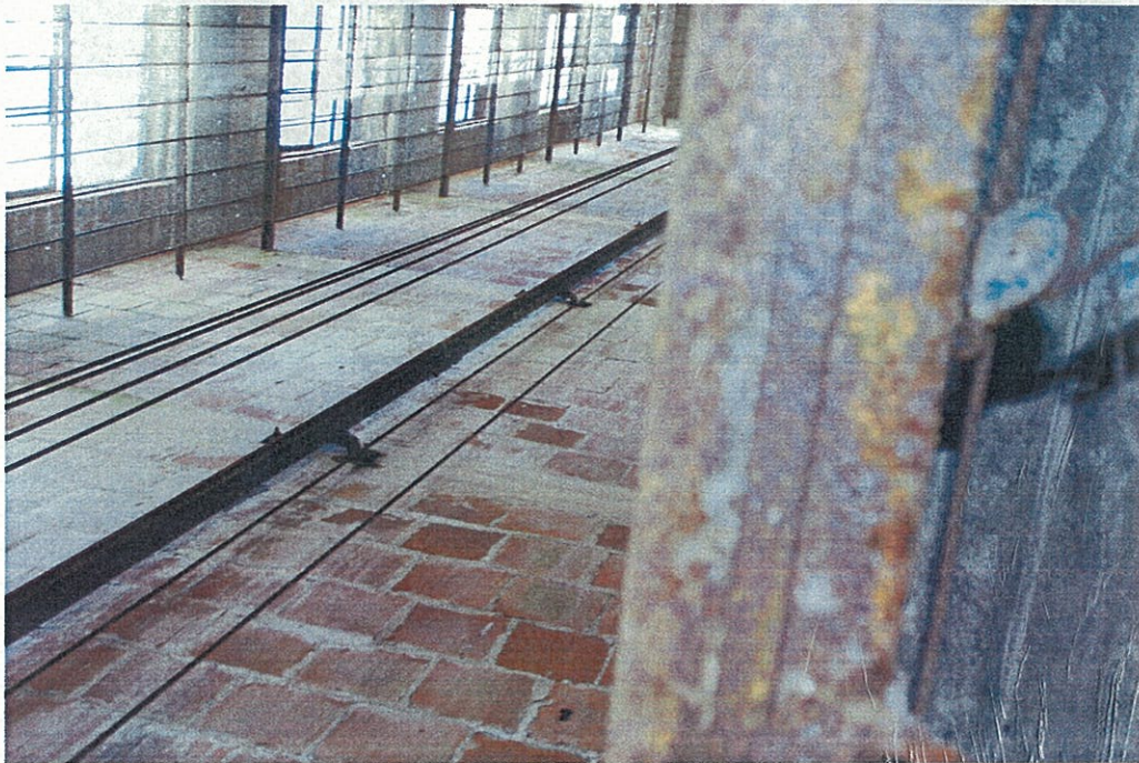
Photo G3.3 – 3 rd Floor
