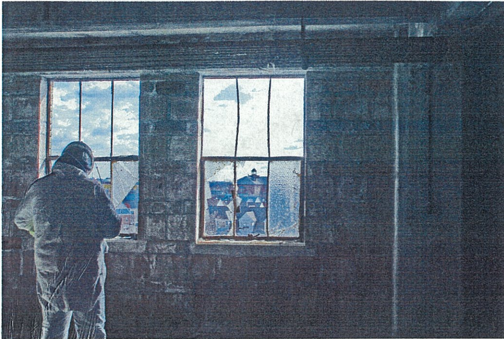
Photo G4.1 – Typical condition for 4 th , 5 th , & 6 th Floors Broken glass and deteriorated window frames.
