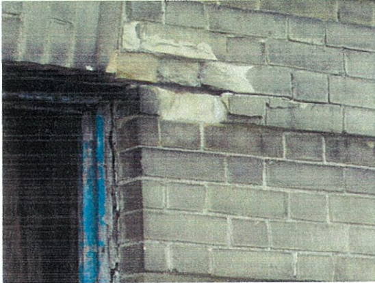
Photo 4: Iron lintel corrosion causing brick spall.
