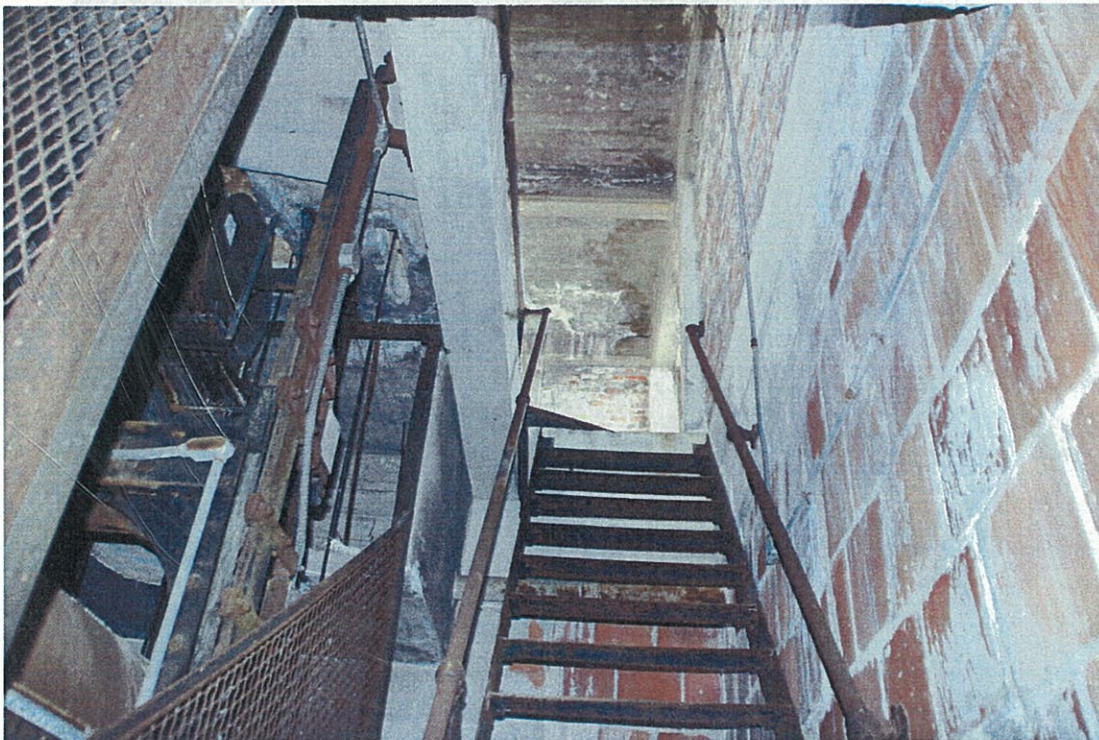
Photo G8.6 – 8 th Floor Highly deteriorated connections along stair leading to building roof.
