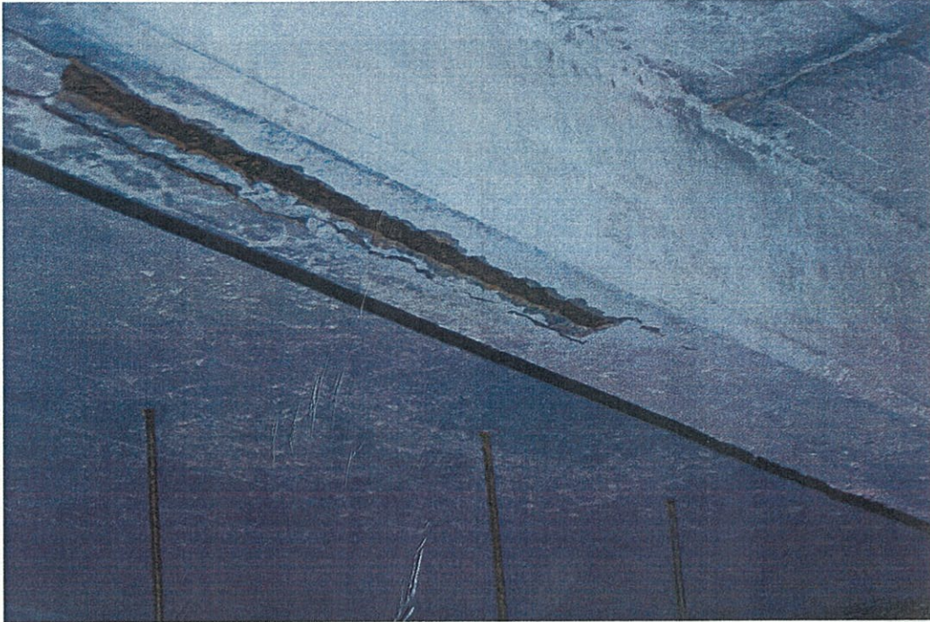
Photo G3.5 – 3 rd Floor Delamination of concrete encasement at underside of beam revealing corrosion of steel section.
