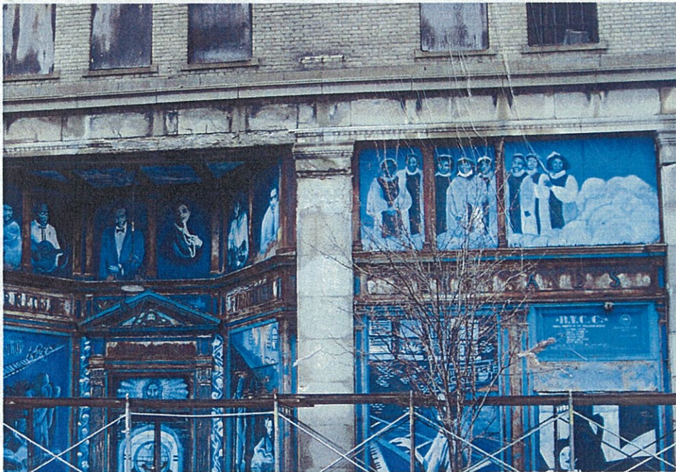
Photo GEX.8 – Front Entrance Scaffolding placed along sidewalk to protect pedestrians from falling debris.
