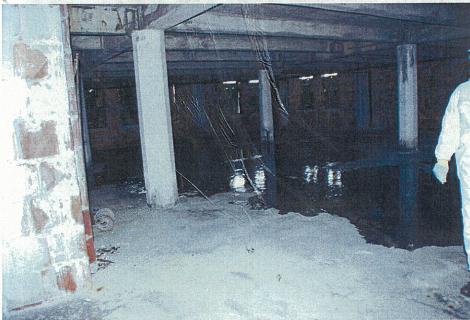
Photo G0.4 - Basement Typical layout of concrete-encased steel columns shown. Large areas of floor covered with ice. Delaminated clay brick walls shown in foreground.
