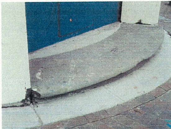
Photo 1: Painted, spalled granite column bases at entry.
