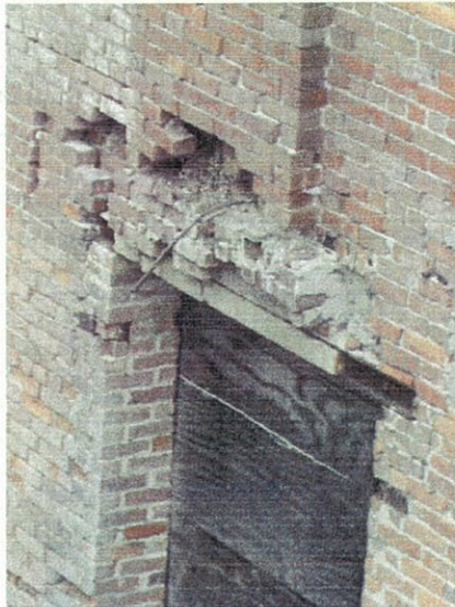
Photo 14: Note loose mortar and brick, brick loss.
