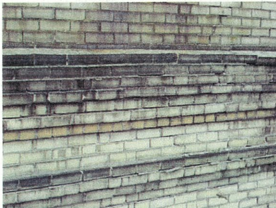
Photo 5: Rust stains, step cracks and open joints at brick.
