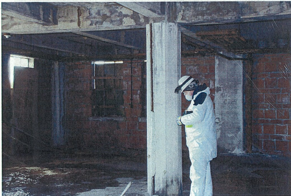
Photo G2.2 – 2 nd (Mezzanine) Floor Delamination and spalling of concrete encasement at column and beams revealing corrosion of steel sections.
