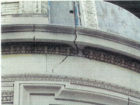
Photo 2: Wide limestone crack at building corner.
