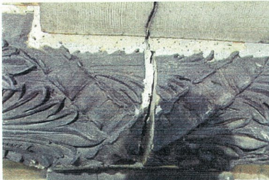
Photo 7: Extremely soiled cream colored terra cotta. Note cracked joint.
