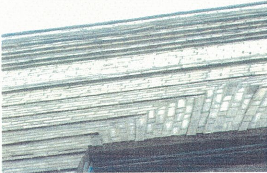
Photo 15: Note bulging courses of brick.
