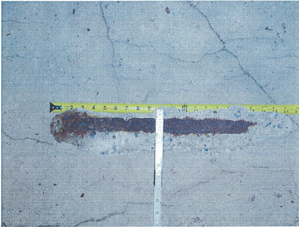
Photo CT0.5 – 5 th Floor Column Concrete sample removed by sledge hammer is 22” x 4”.
