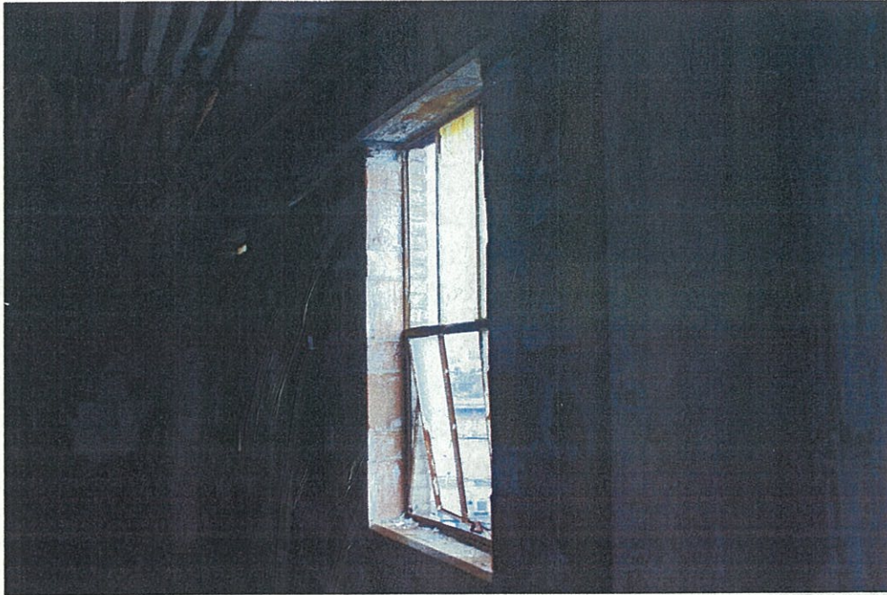
Photo G8.3 – 8 th Floor Broken glass and deteriorated window frame.
