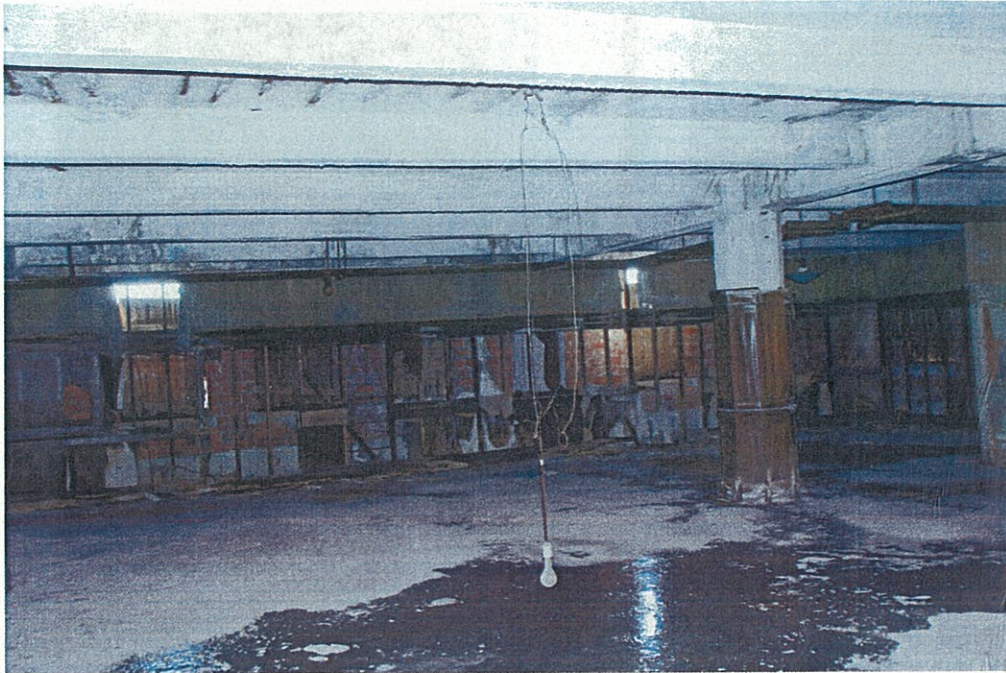
Photo G2.1 – 2 nd (Mezzanine) Floor Exposed abandoned utilities and showroom wood work on walls and columns shown. Floor covered with ice and fallen plaster.
