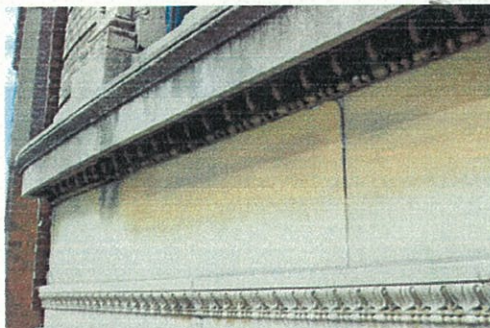
Photo 3: Rust stains on limestone.
