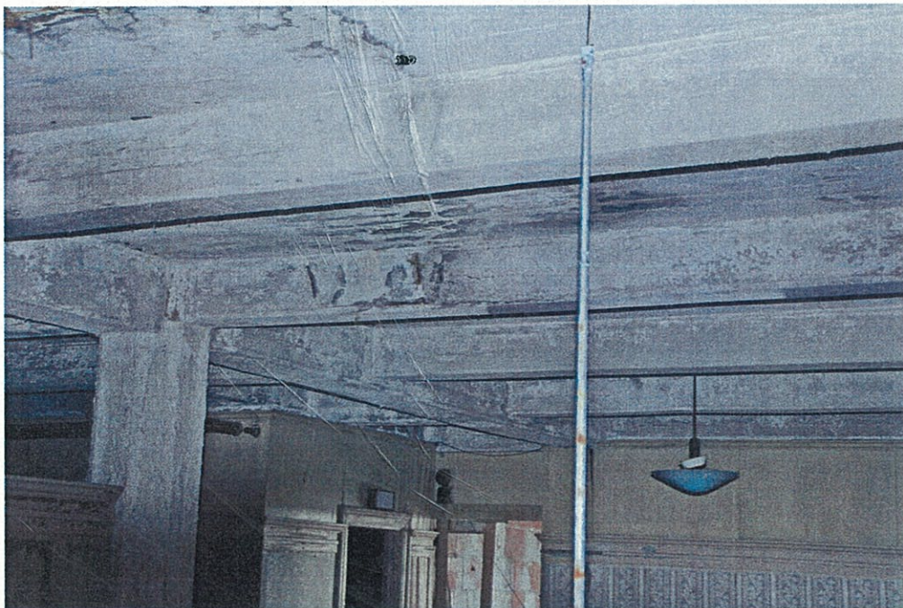
Photo G5.2 - 5 th Floor Spalling at underside of 6 th floor slab and concrete-encased steel beams. Water stains follow apparent conduit to fixtures and junction boxes.
