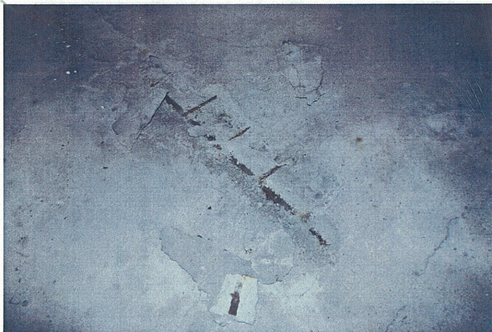
Photo G6.2 – 6 th Floor Exposed corroded reinforcement in concrete floor.
