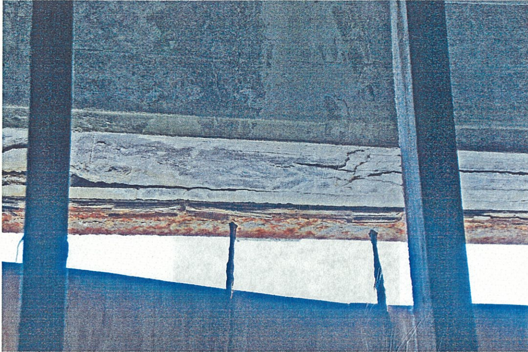
Photo G4.3 – 4 th Floor Deteriorated concrete around window lintels.
