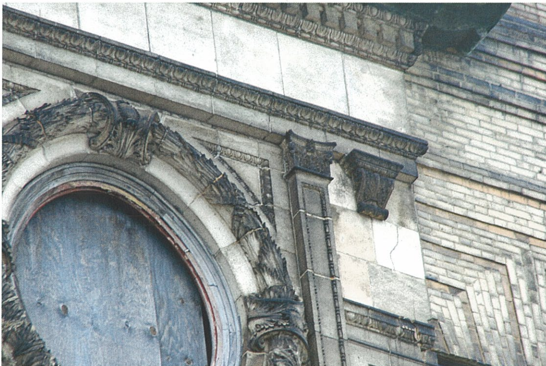
Photo FEX.7 – Building Exterior Crack in façade near window.
