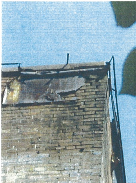
Figure 4: Ferdinand Building - Warren Street Elevator Shaft Widespread loss of mortar
