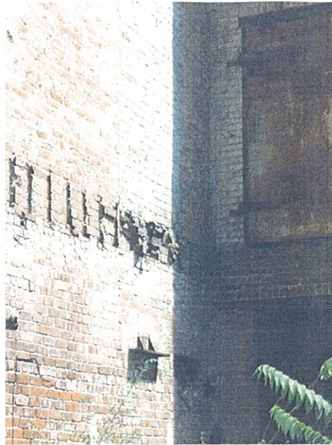
Figure 5: Ferdinand Building - Warren Street Elevator Shaft Apparent "soft" joint between shaft and building
