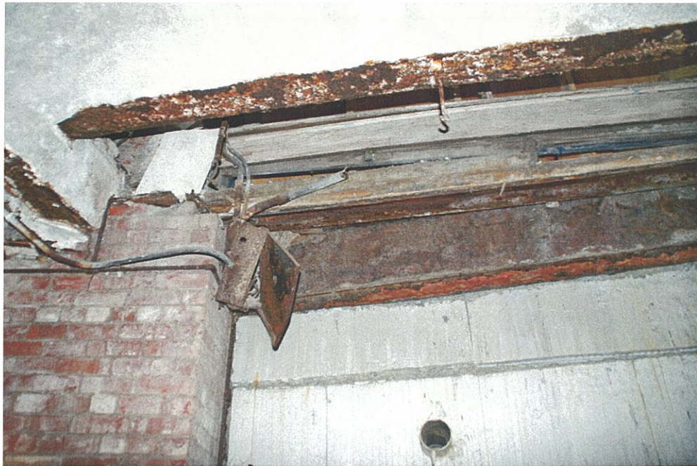
Photo F0.3 - Basement Exposed, deteriorated steel framing at the opening in the 1 st Floor concrete slab.
