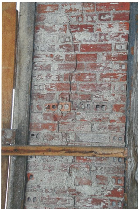
Photo F3.1 – 3 rd Floor Cracking in brick pilaster located between Warren Street windows.
