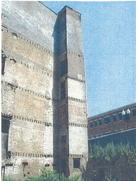
Figure 1: Ferdinand Building - Warren Street Elevator Shaft Elevation view as seen from vacant lot
