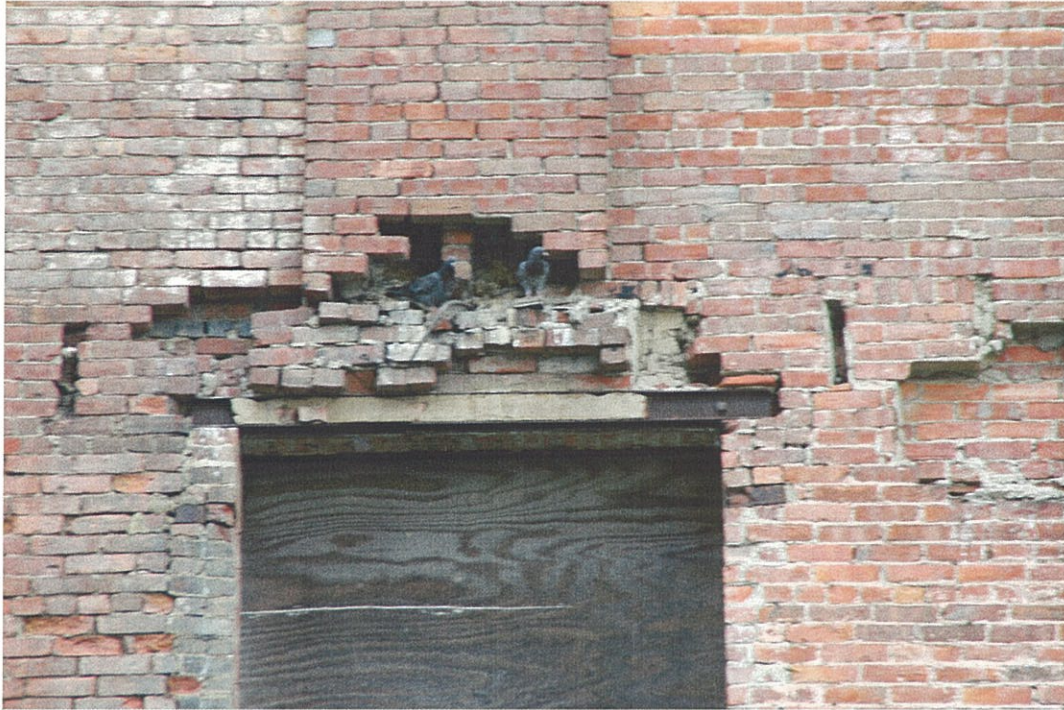
Photo FEX.6 – Building Exterior Brick chimney on south façade – significant brick deterioration.
