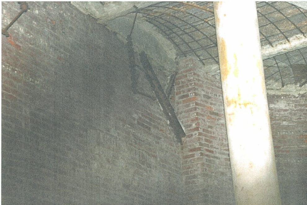
Photo F5.10 – 5 th Floor Fallen plaster from arched ceiling reveals curved reinforcing bars. Diagonal bracing to brick pilaster can also be seen.
