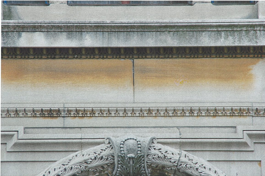
Photo FEX.10 – Building Exterior Cracking observed in stone.
