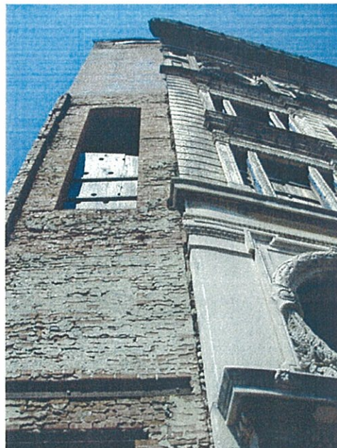
Figure 2: Ferdinand Building - Warren Street Elevator Shaft Elevation view as seen from Warren Street
