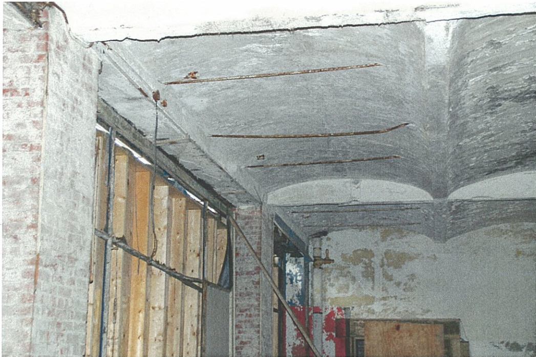
Photo F3.3 – 3 rd Floor Deterioration in arched plaster ceiling.
