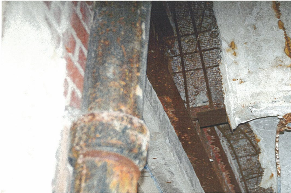
Photo F1.3 – 1 st Floor Looking up at connection between floor structure and exterior wall.
