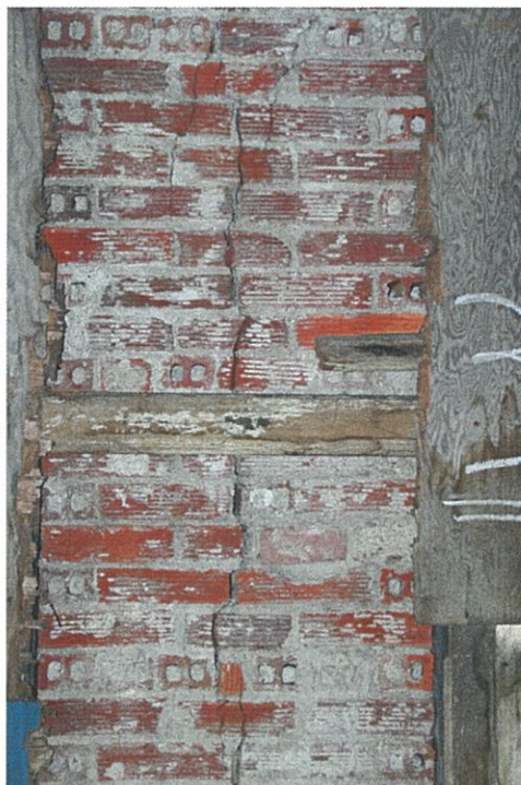
Photo F3.2 – 3 rd Floor Cracking in brick pilaster located between Warren Street windows.
