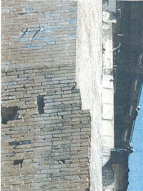
Figure 3: Ferdinand Building - Warren Street Elevator Shaft Widespread loss of mortar
