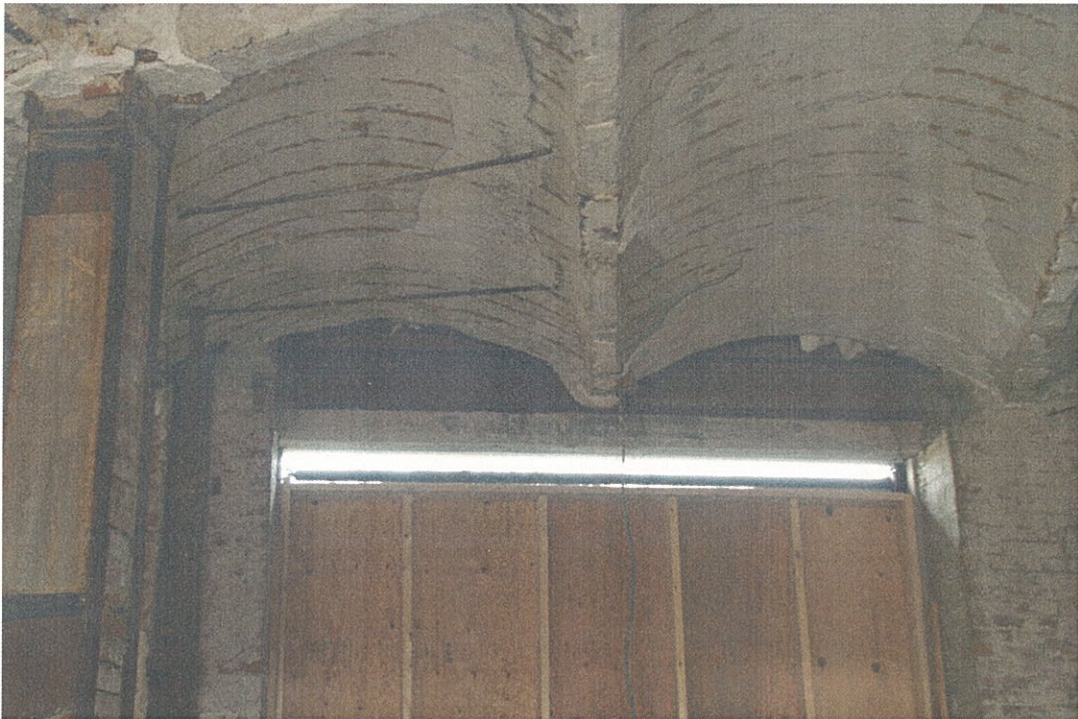
Photo F5.5 – 5 th Floor Deterioration at arched plaster ceiling and roof framing.
