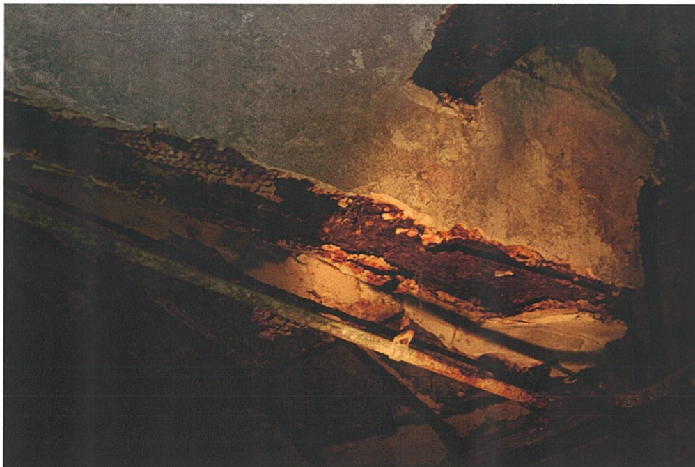
Photo F0.4 - Basement Delamination and spalling of concrete at underside of floor beam revealing corrosion of steel section.
