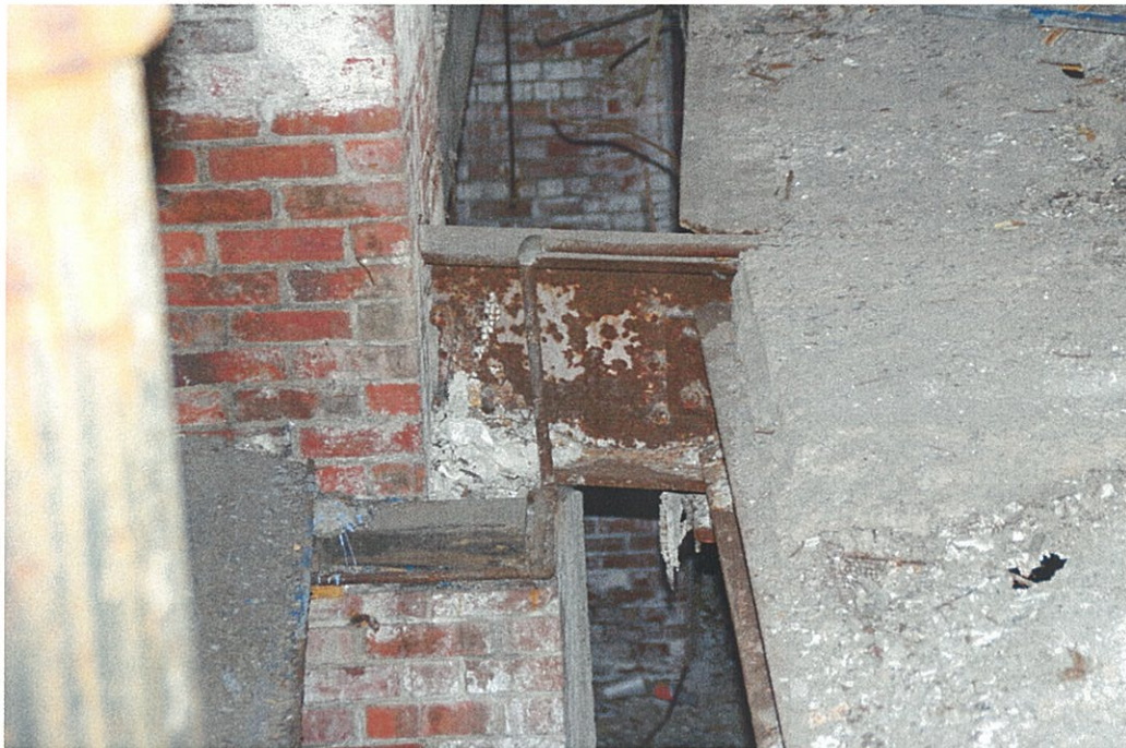
Photo F1.1 – 1 st Floor 1 st Floor slab opening and connection between floor structure and exterior wall.
