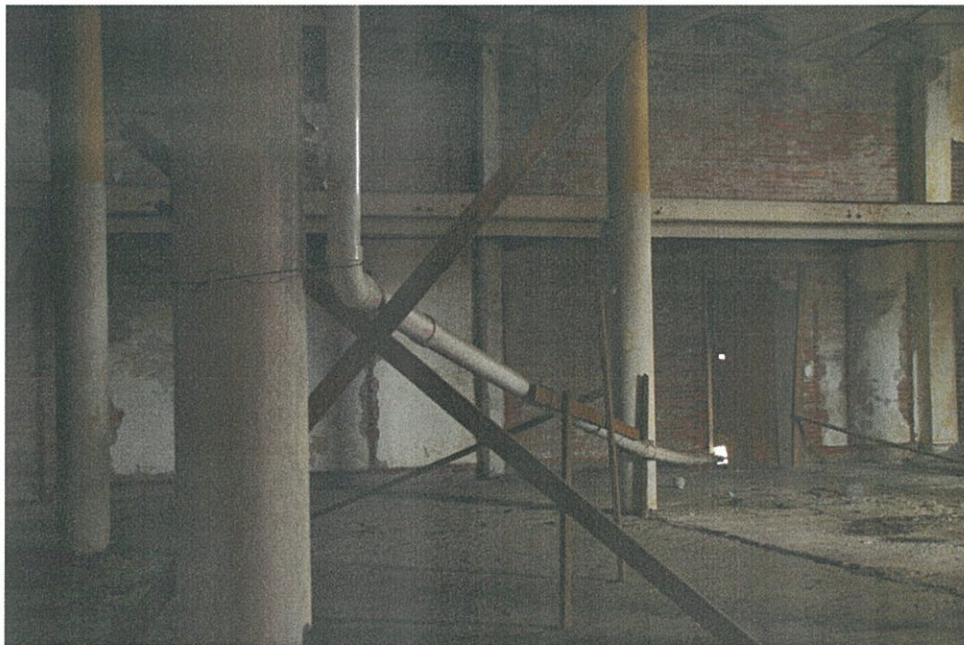
Photo F5.6 – 5 th Floor Elevation showing roof scupper drainage system and mezzanine level beyond.
