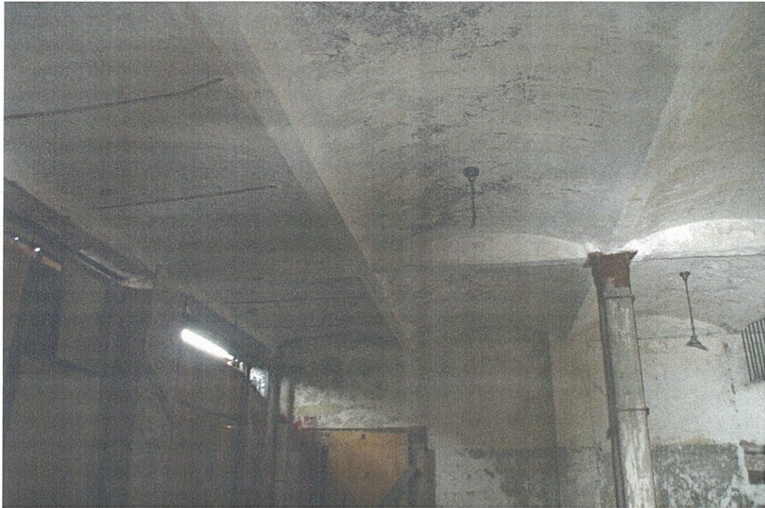
Photo F4.1 – 4 th Floor General interior elevation and typical structural framing system.
