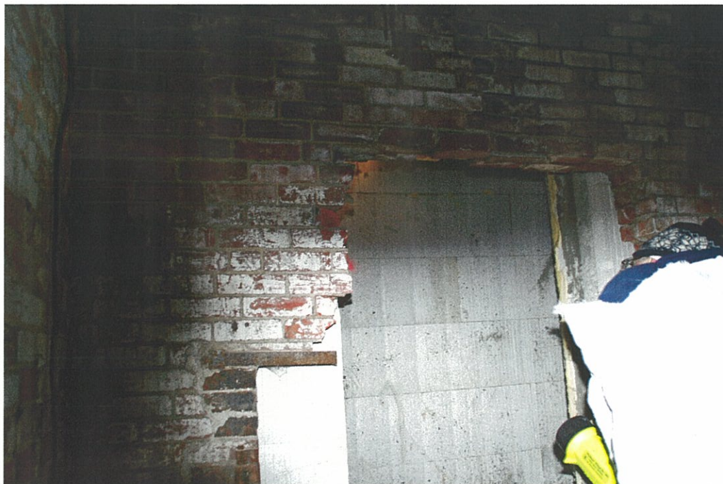
Photo F0.6 - Basement Electric vault.
