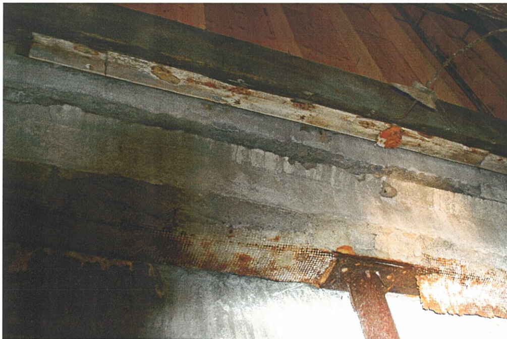
Photo F0.2 - Basement Connection between lally column and concrete-encased steel beam at the opening in the 1 st Floor concrete slab.
