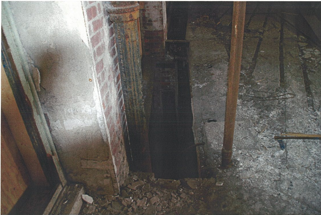
Photo F2.3 – 2 nd Floor Elevation at window base and adjacent brick pilaster.
