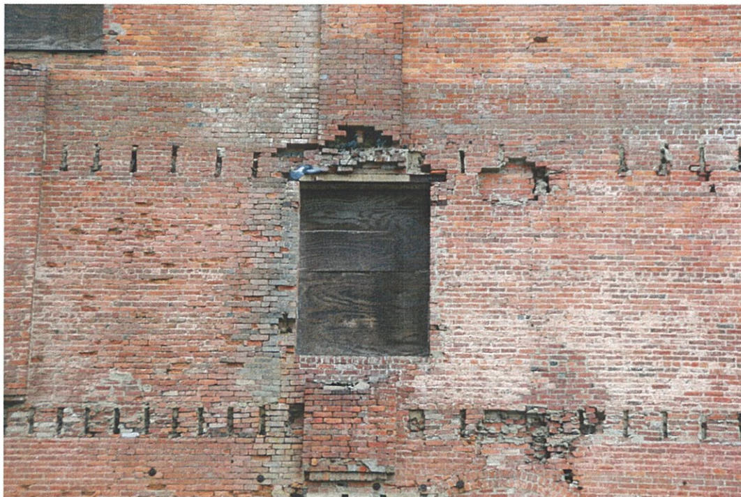
Photo FEX.5 – Building Exterior Brick chimney on south façade – significant brick deterioration.
