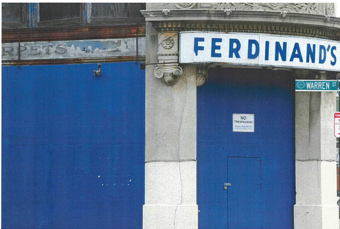
Photo FEX.9 – Building Exterior Crack in masonry columns at building entrance.
