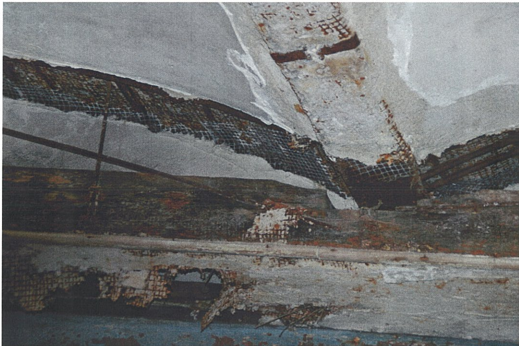
Photo F1.9 – 1 st Floor General deterioration at interface of floor structure underside and exterior wall.
