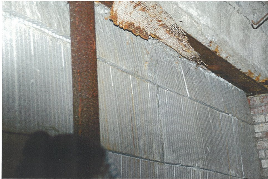
Photo F0.1 - Basement Lally column near the opening in the 1 st Floor concrete slab.
