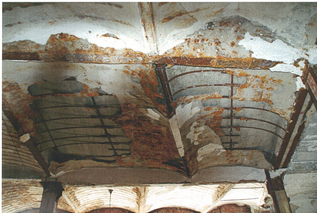
Photo F3.4 – 3 rd Floor Fallen plaster from arched ceiling reveals curved reinforcing bars.
