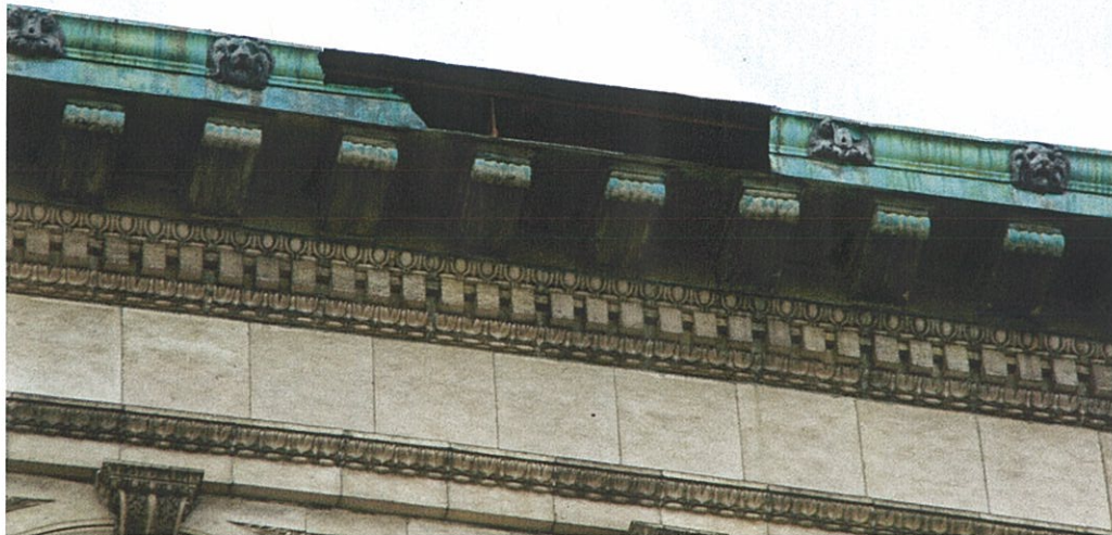
Photo FEX.11 – Building Exterior Portion of cornice missing.
