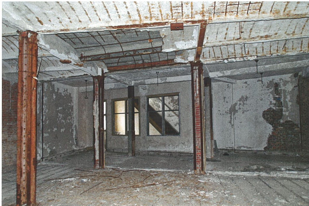
Photo F2.2 – 2 nd Floor General interior elevation and typical structural framing system.
