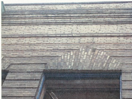
Figure 10. Bowing brick courses at addition.
