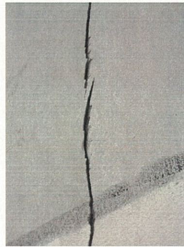
Figure 4. Shear crack in limestone.
