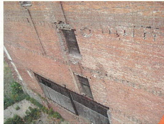
Figure 11. South elevation brick deterioration.
