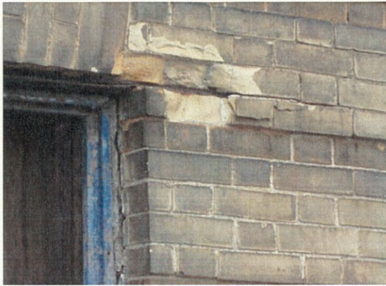
Figure 8. Spalled brick at site of iron corrosion/expansion.
