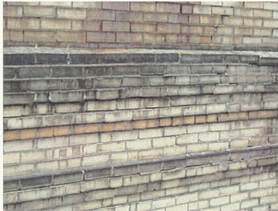
Figure 26. Cracked and open brick joints.
