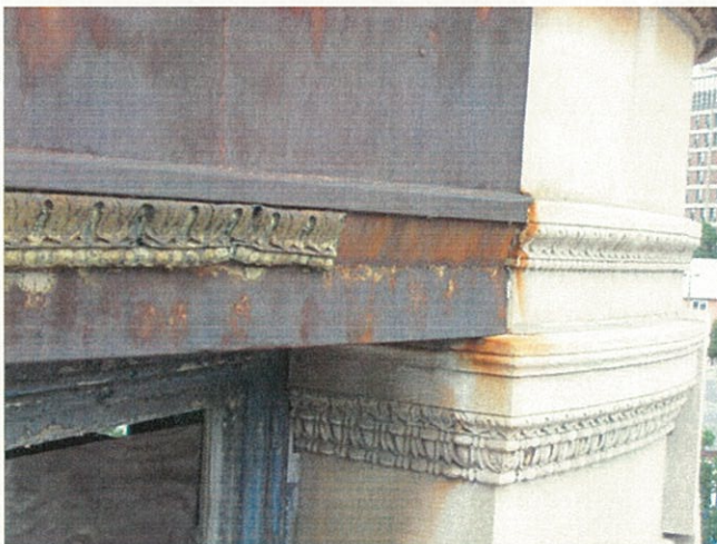
Figure 5. Rust staining at limestone column.
