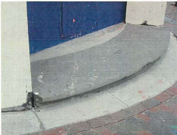
Figure 18. Granite spalls at main entry, building corner.
