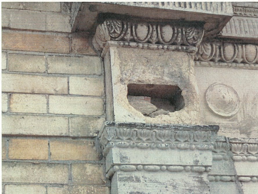
Figure 16. Large spall in terra cotta.
