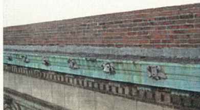
Figure 12. The brick parapet wall above the cornice was formerly covered in copper. It is in good condition.
