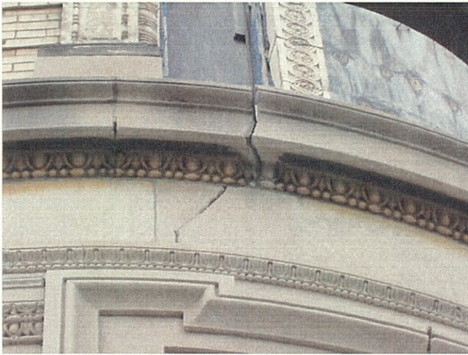
Figure 3. Wide crack in limestone at building corner.
