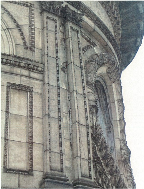
Figure 15. Bowing terra cotta units in right pilaster.
