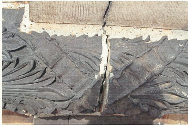
Figure 14. Extreme soiling and soot deposition on cream-colored terra cotta.
