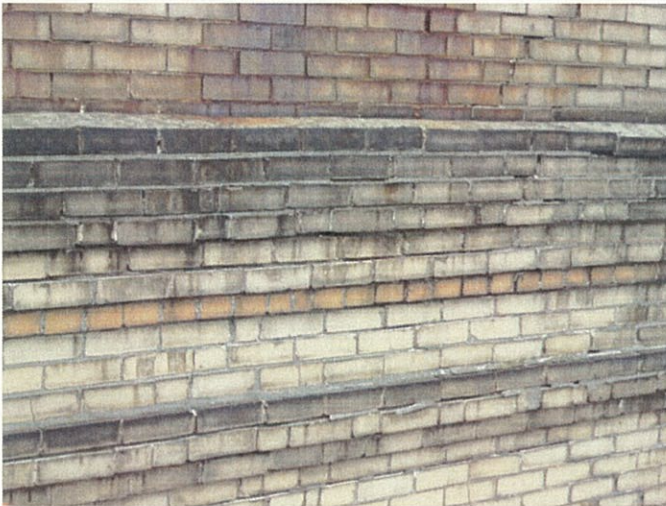
Figure 6. Soiling, open joints, cracked joints and staining at brick.
