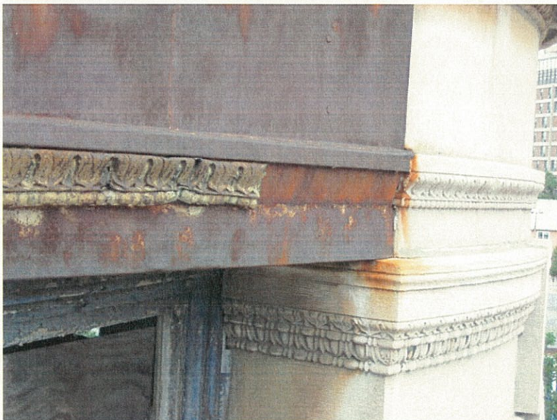
Figure 22. Corroding metal trim has stained limestone at first floor.
