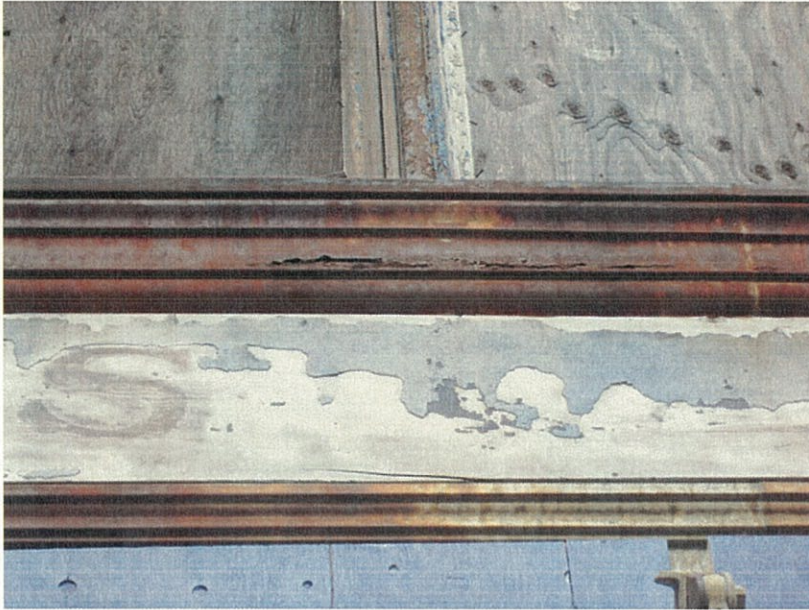
Figure 21. Deteriorated ferrous metal trim.
