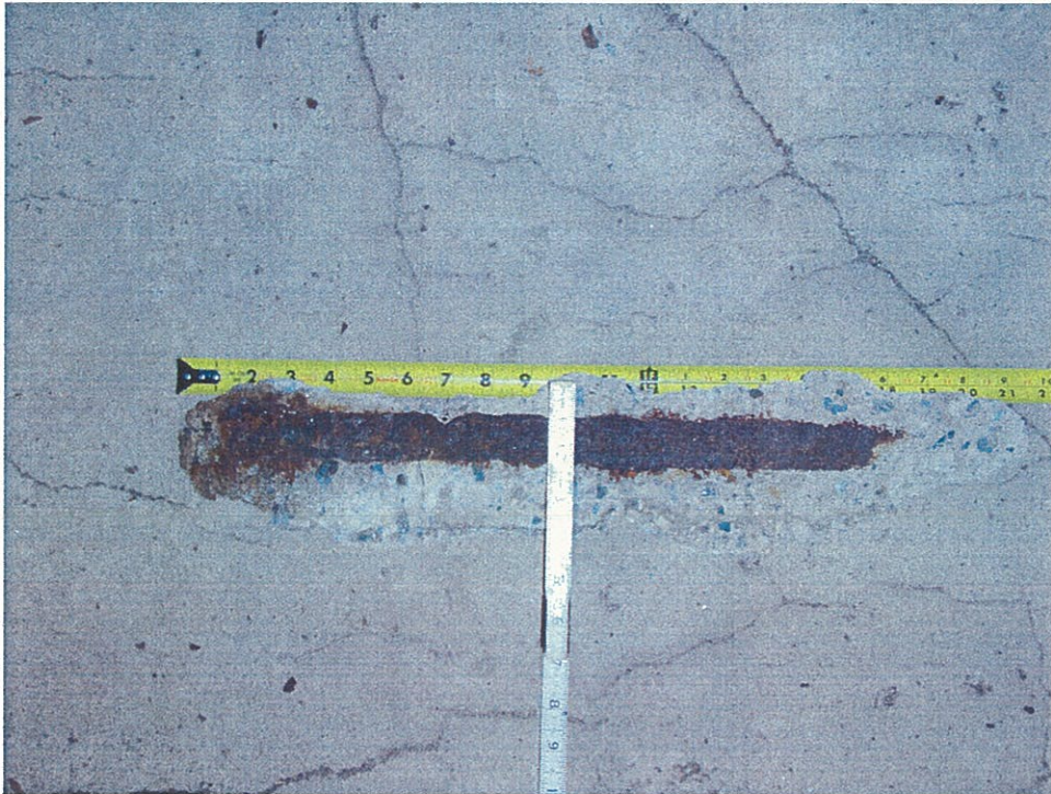
Photo CT0.5 – 5 th Floor Column Concrete sample removed by sledge hammer is 22” x 4”.
