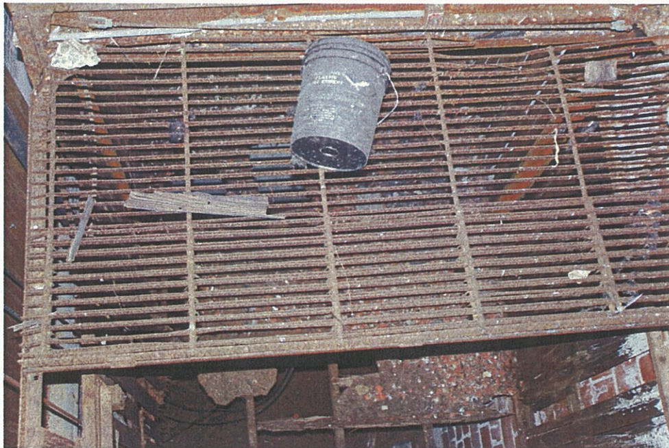
Photo G3.4 – 3 rd Floor
