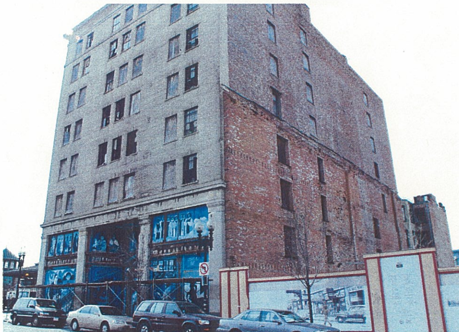
Photo GEX.2 - Elevation Picture taken from vacant lot opposite side of Warren Street gate. Scaffolding placed along sidewalk to protect pedestrians from falling debris. Deteriorated glass and window frames can be observed.
