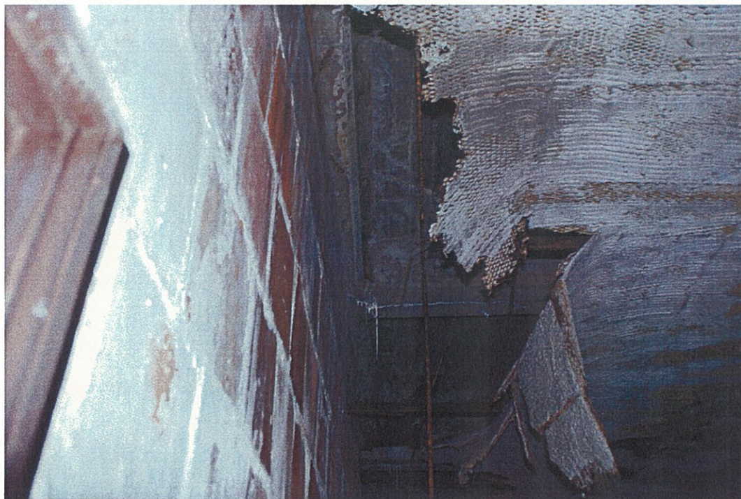
Photo G8.4 – 8 th Floor Ceiling deterioration at exterior walls.
