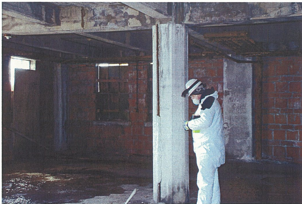
Photo G2.2 – 2 nd (Mezzanine) Floor Delamination and spalling of concrete encasement at column and beams revealing corrosion of steel sections.
