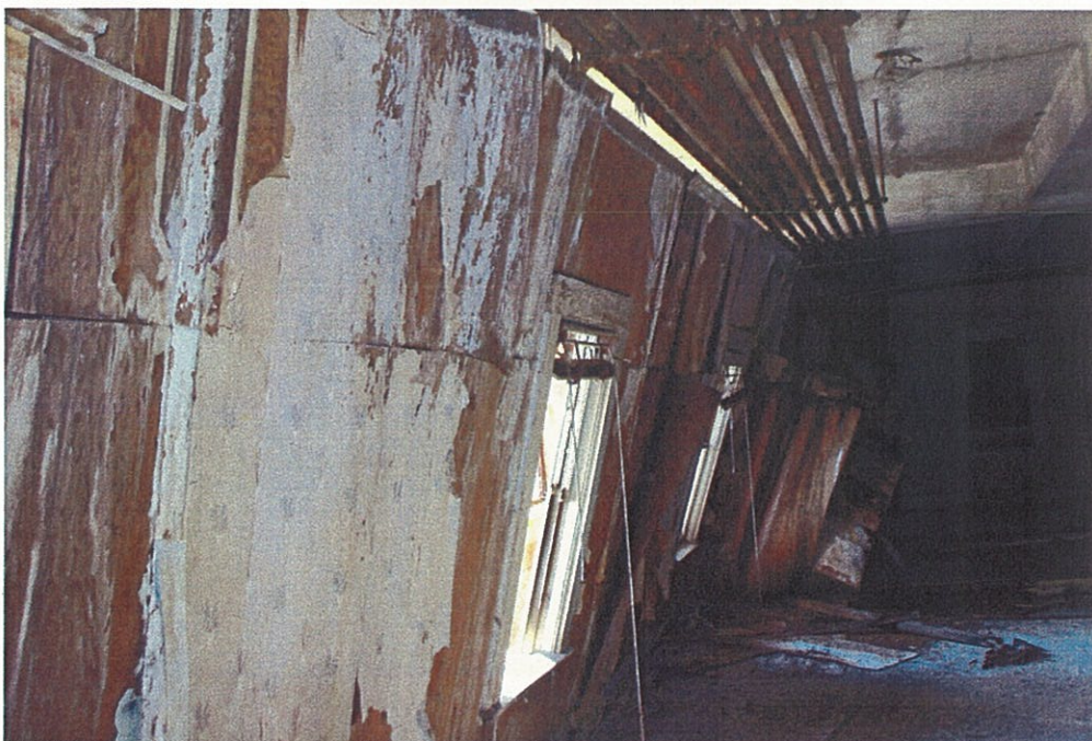
Photo G4.4 – 4 th Floor Unstable wall partitions ready to fall.
