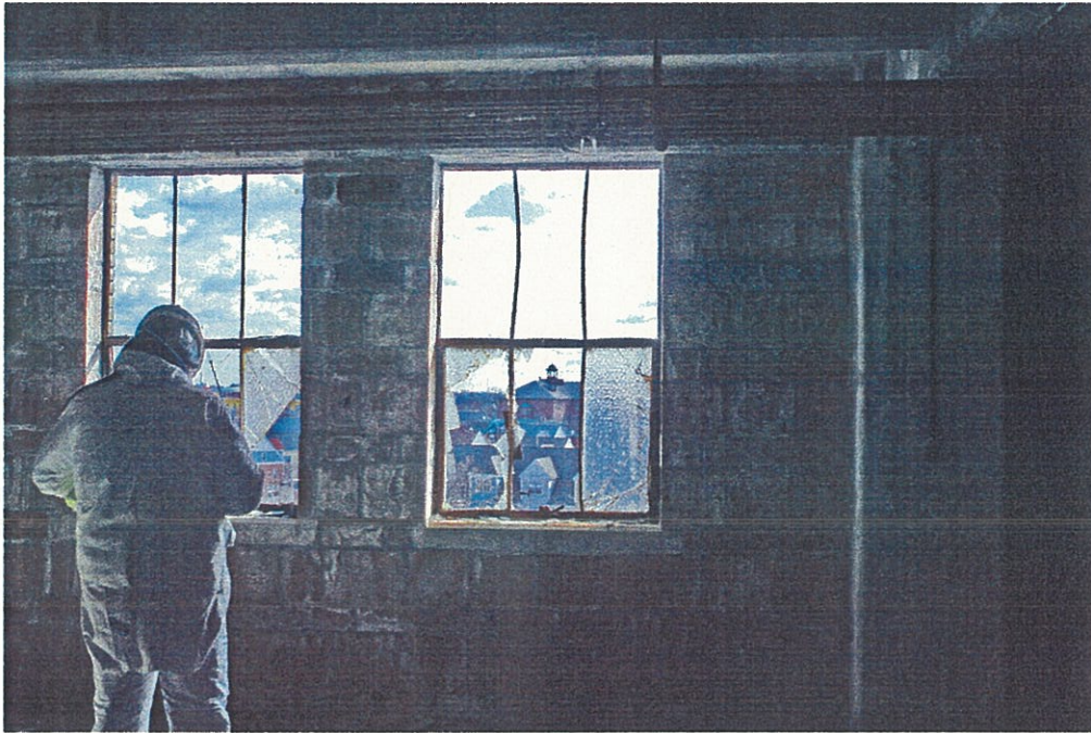
Photo G4.1 – Typical condition for 4 th , 5 th , & 6 th Floors Broken glass and deteriorated window frames.
