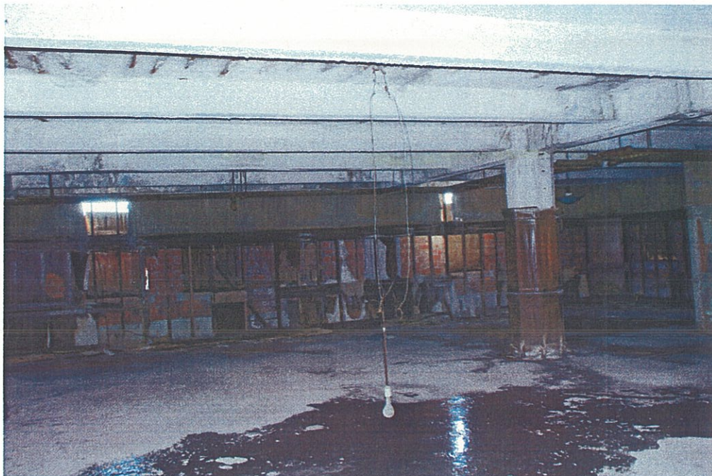
Photo G2.1 – 2 nd (Mezzanine) Floor Exposed abandoned utilities and showroom wood work on walls and columns shown. Floor covered with ice and fallen plaster.
