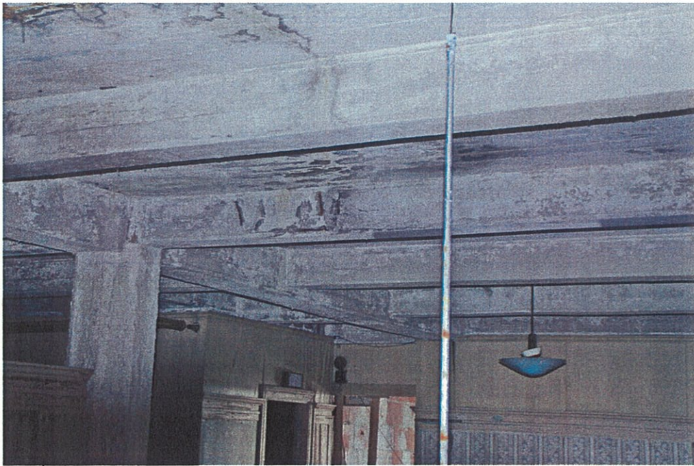
Photo G5.2 - 5 th Floor Spalling at underside of 6 th floor slab and concrete-encased steel beams. Water stains follow apparent conduit to fixtures and junction boxes.
