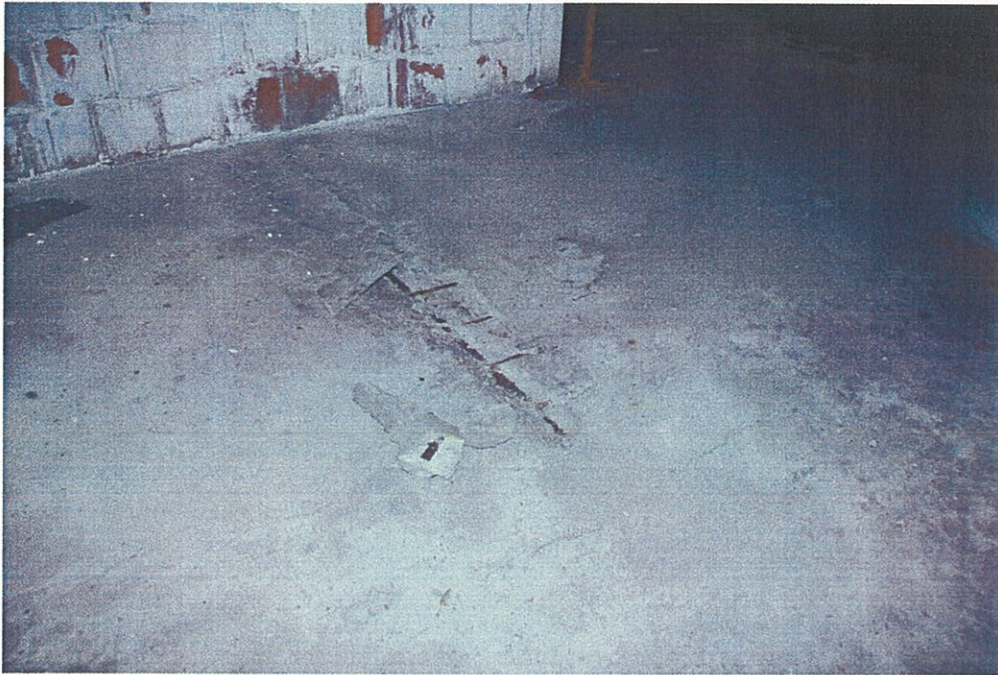
Photo G6.1 – 6 th Floor Exposed, corroded reinforcement in concrete floor.
