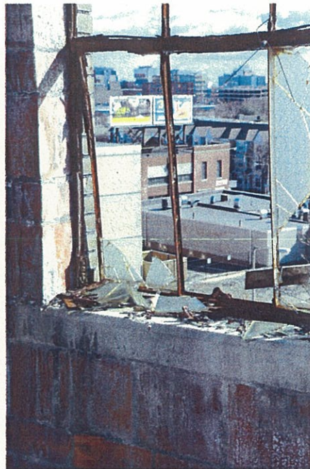
Photo G4.2 – Typical condition for 4 th , 5 th , & 6 th Floors Broken glass and deteriorated window frames.
