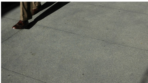
Sidewalk with darker grey color, smooth finish, saw-cut joints, and dark surface aggregate.
