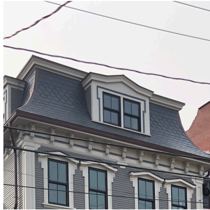
Roof forms, such as this Mansard Roof, contribute to the overall visual character of a block, especially when they utilize changes in depth and material.
