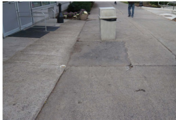
pavement in poor condition
