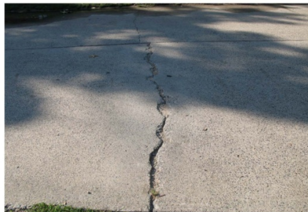
significant pavement cracks
