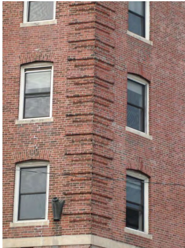
Detail of quoins at the corner of Mass. Ave and Belvidere Ave.
