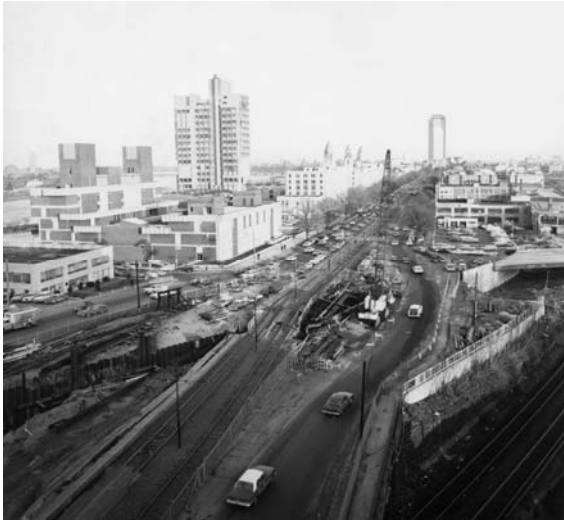
Figure 4-15, Massachusetts Turnpike and Commonwealth Avenue during construction of the Carlton Street Overpass
