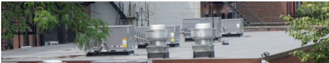
Fisher Mall Roof Showing 4 HVAC systems and 2 Exhaust Stacks
