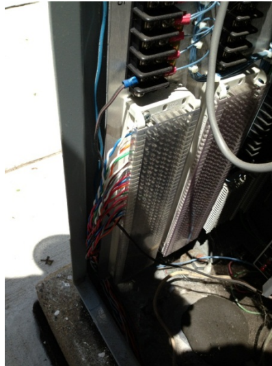
Existing In-Cabinet Interconnect Cable - North Harvard Street/Easton Street
