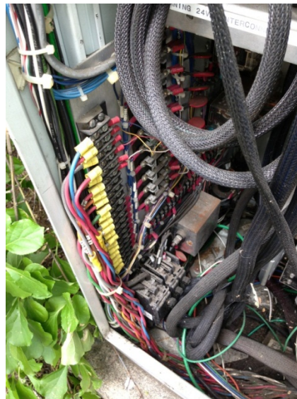
Existing In-Cabinet Interconnect Cable - Cambridge Street / Window Street
