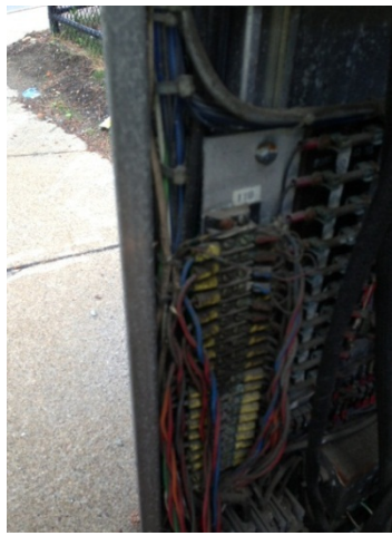
Existing In-Cabinet Interconnect Cable - Cambridge Street / North Harvard Street
