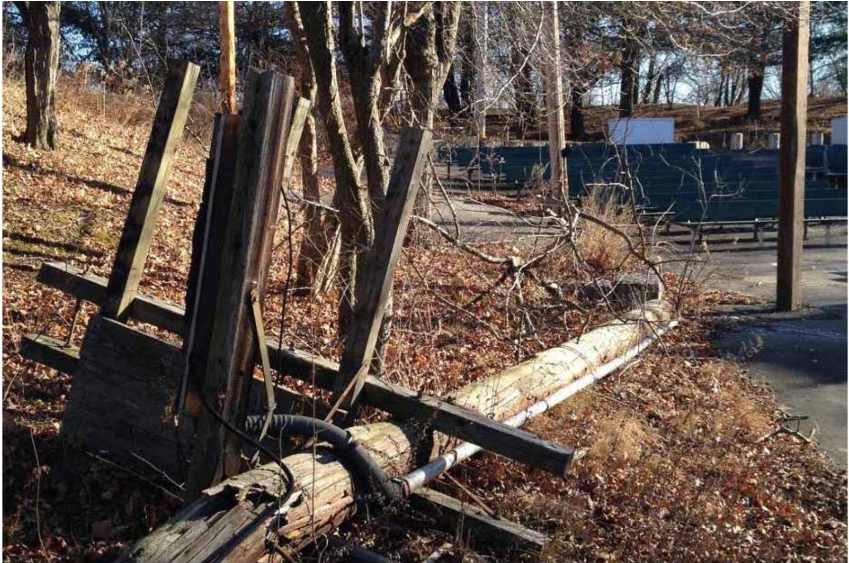
Downed utility poles & power lines pose a public safety hazard.
