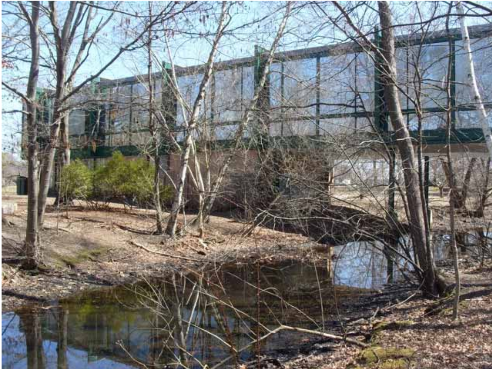
The moat is silted in & clogged with debris. Invasive species of plants have overtaken the banks. The Herter Center is showing signs of advanced decay.
