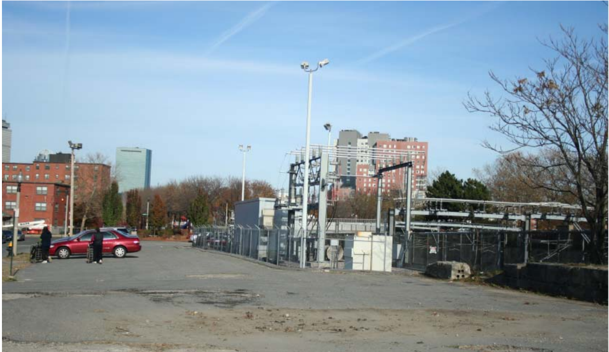
Figure 16: Amtrak Installation on Mindoro Lot
