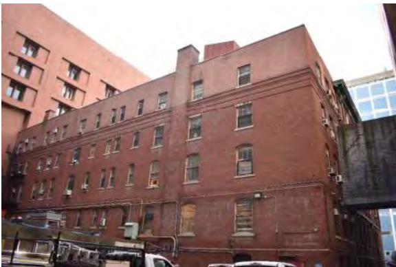
3. Back of Vose Hall (northeast elevation) with elevated walkway to the Robinson Building (on right).
