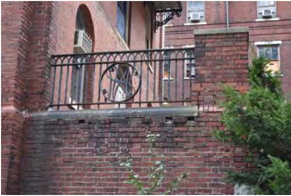
1. Area of missing and displaced brick under cast iron railing. Area also shows deteriorated and open joints.
