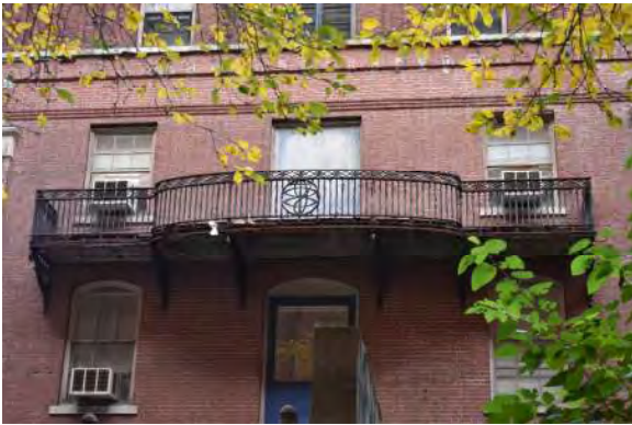
3. Original cast iron balcony with some deterioration.
