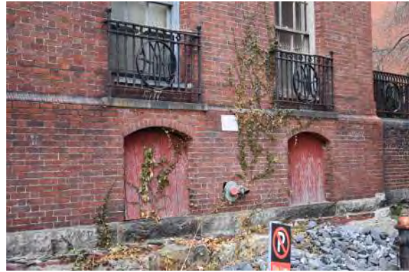
2. Deteriorating paint and wood board over basement windows, along with soiling on limestone and granite and vegetation growing on brick wall.
