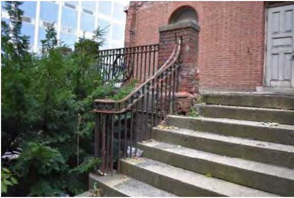
1. Cast iron railing is in poor condition and the brick pier has significant mortar loss and rust jacking.
