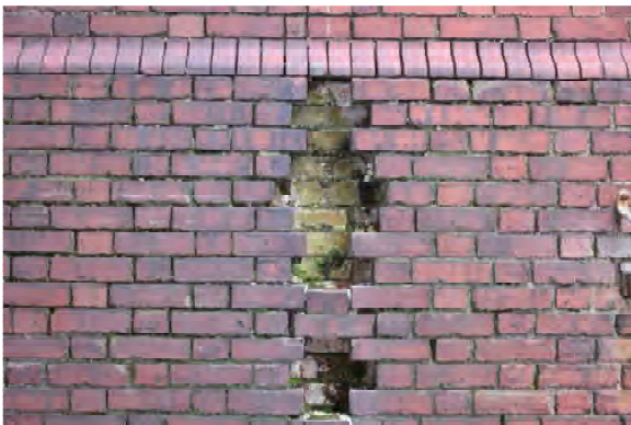
3. Area of missing brick and deteriorated mortar joints.
