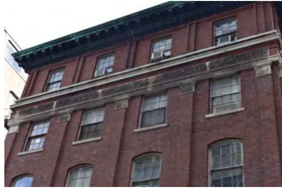
2. Limestone inscription band is in good condition despite heavy soiling. Copper cornice above is missing components and has open seams.
