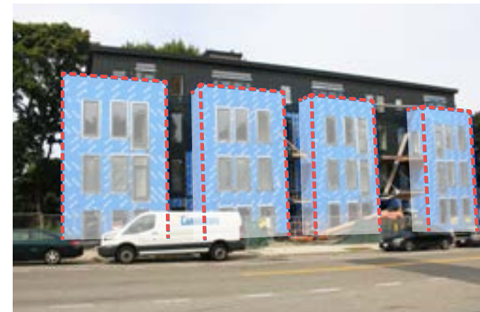
Article 80 project under construction at 59-63 Belgrade Avenue, which includes 3-story bays to minimize scale
