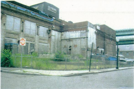
View looking west across the northeast elevation of building showing partial demolition.
