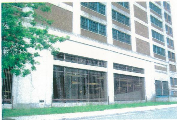
View looking west at northeast elevation. Note loading dock infill and window treatments.
