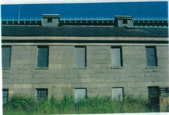
View of a portion of the Ropewalk showing restored cupolas, repaired slate roof, covered skylights, rebuilt brick eave detail and three generations of window coverings.
