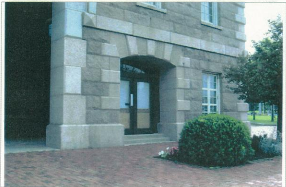
First floor detail of southwest elevation looking east. Note replacement windows and recessed doors.
