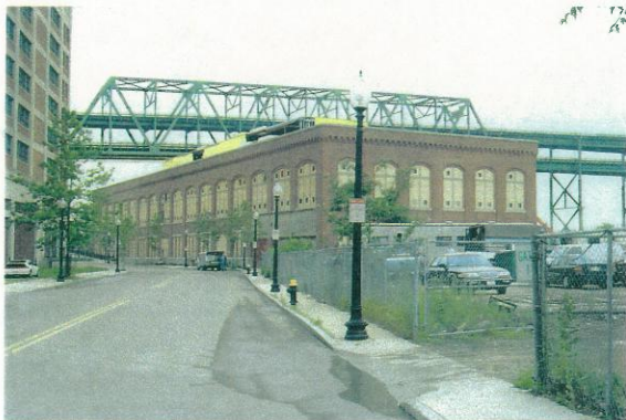
View looking northwest along Sixteenth Street showing rehabilitation in progress on Building 114.
