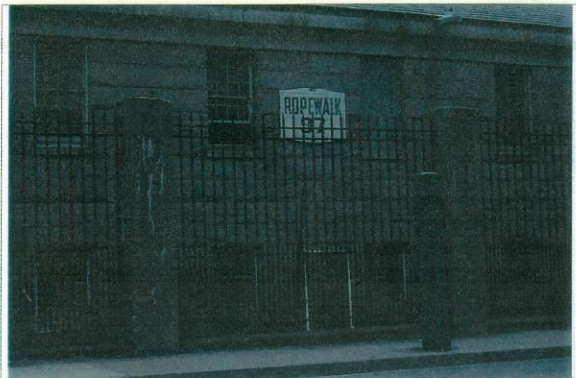
Detail view of northeast elevation showing metal screening and plywood enclosures at windows. 7/16/00
