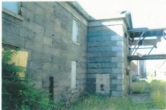
Detail looking south at entrance pavilion on northwest elevation. Note stabilized bridge connecting to the Ropewalk Building. 7/21/00
