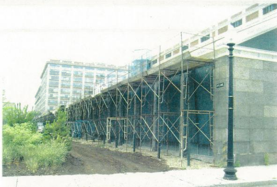
View looking west along Second Avenue. Scaffold is in place for roof replacement.
