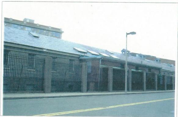
View looking south from Chelsea Street showing 20th century brick addition to Ropewalk.
