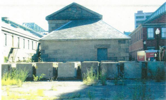
View looking northeast at southwest addition which required significant roof and masonry repairs.
