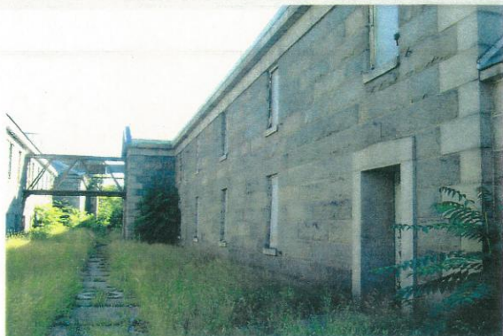
View looking east at northwest elevation showing proximity to the Ropewalk Building. 7/21/00
