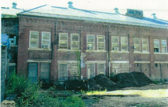
View looking southeast at the easterly portion of the northeast elevation where low buildings were removed at the link with Building 108.
