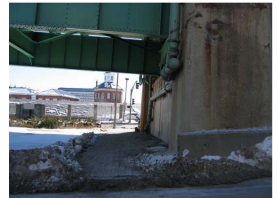
This pedestrian connection under the Tobin Bridge overpass, as well as an additional tunnel connection at Gate 1 are main routes to the Navy Yard from uptown Charlestown. These two connections lack signage, lighting and a friendly design to encourage use and welcome Charlestown residents to the Yard.
