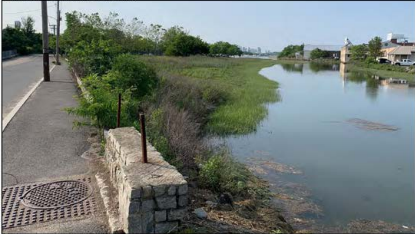
Photo 2: View of Pine Neck Creek, and existing retaining wall, and the salt marsh along the edge of Tenean Street.
