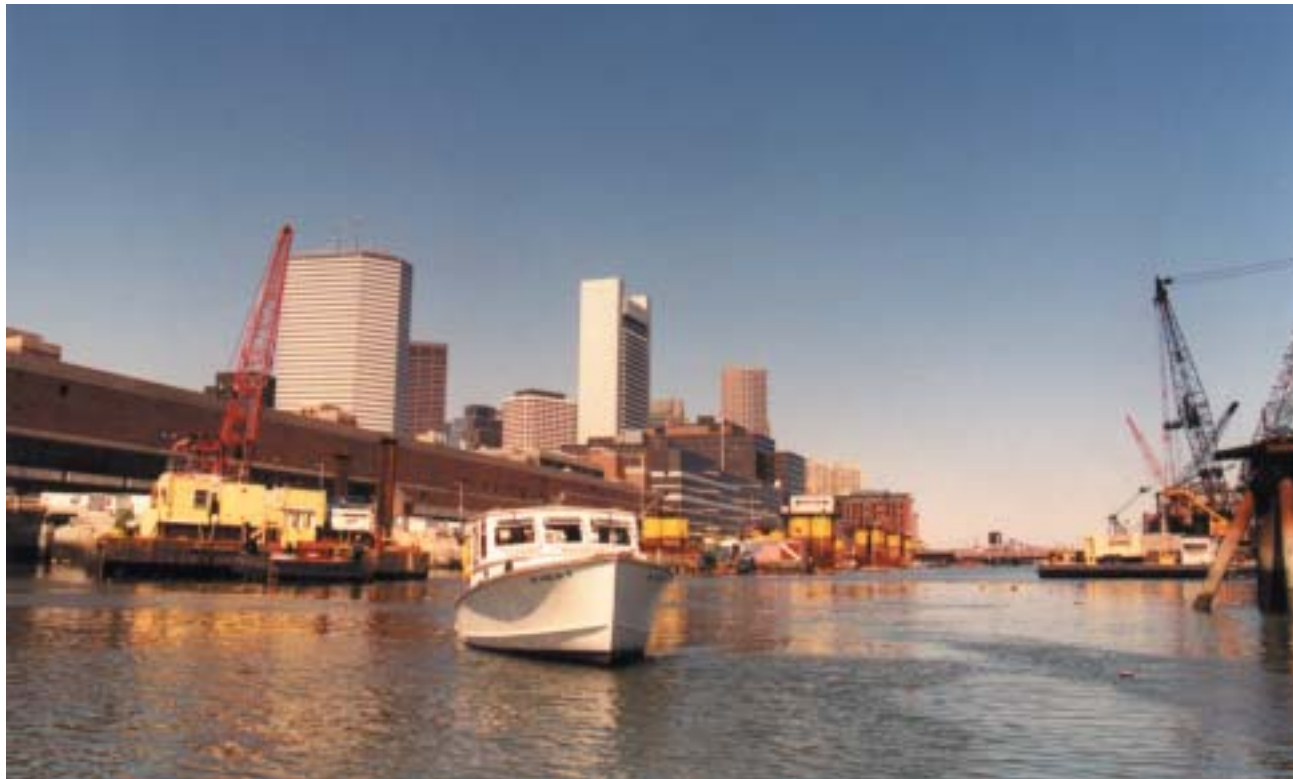
The Fort Point Channel watersheet with construction underway in 2001. This underutilized waterway presents an opportunity to create a unique public space in the heart of the city.
