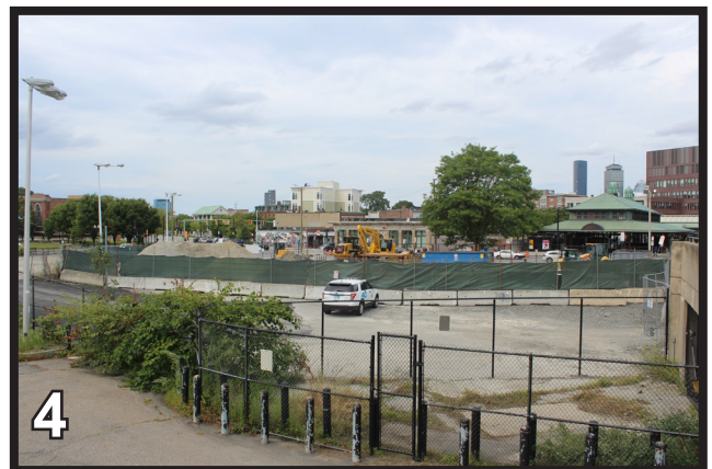
View of the Project Site from the Roxbury Municipal Court looking North
