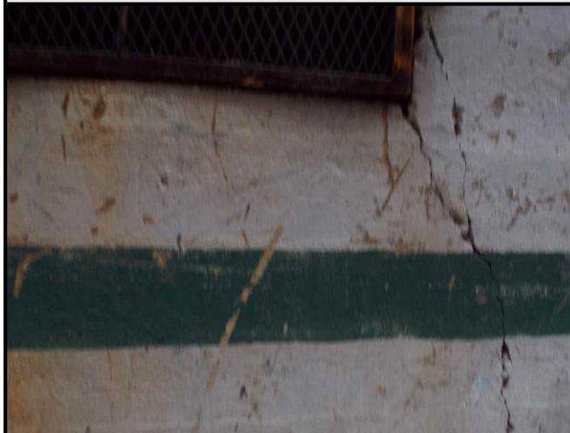
Cracked foundation wall
