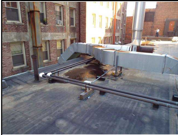
Ponding on "L" roof
