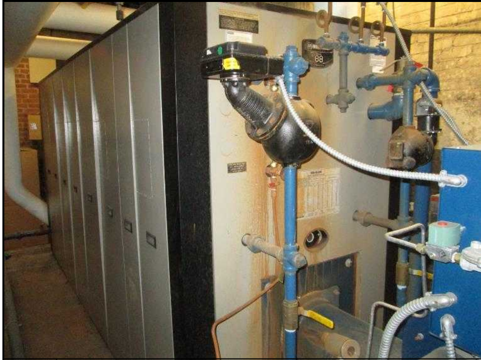
31. Gas fired boiler
