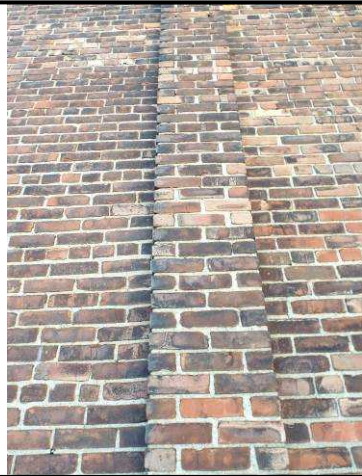
Brickwork requiring minor repointing
