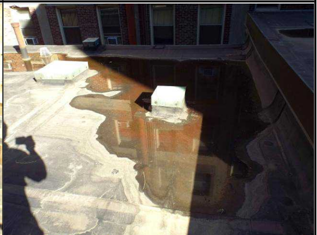
Ponding on "L" roof
