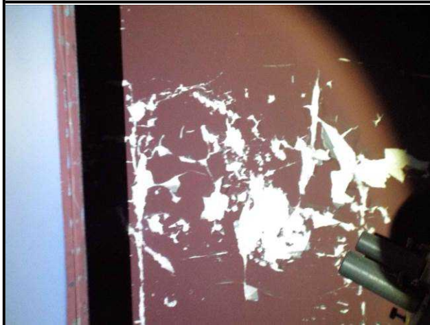
Location of additional drain failure
