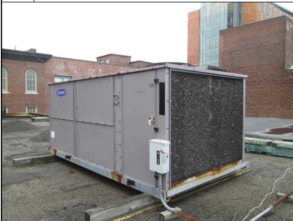
12. 252 Huntington rooftop HVAC unit
