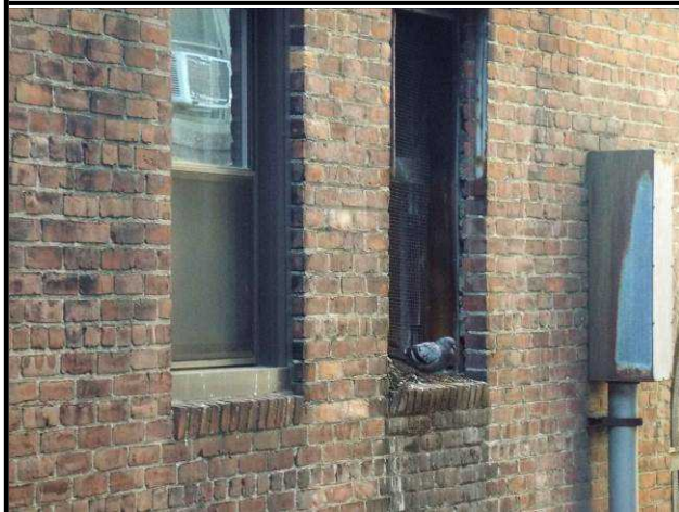
Failed sealants at windows
