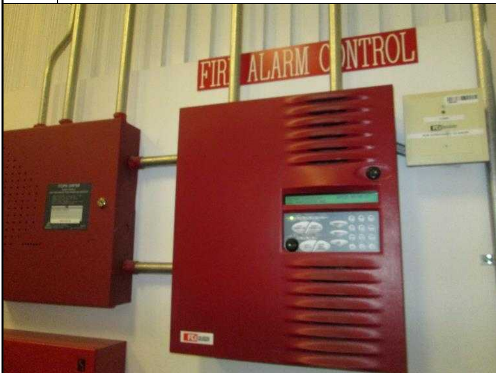
26. 252 Huntington fire alarm control panel
