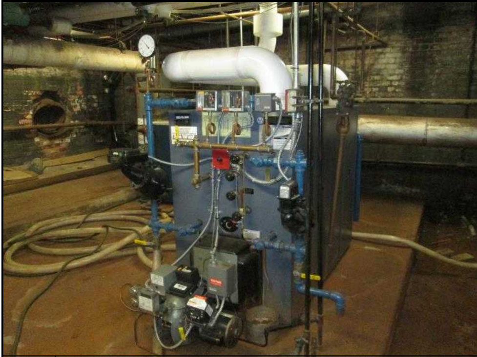
35. 258 Huntington oil boiler
