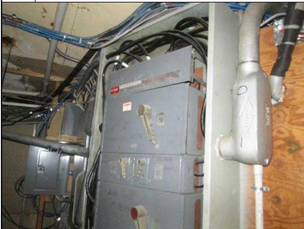
30. 252 Huntington electrical switchgear
