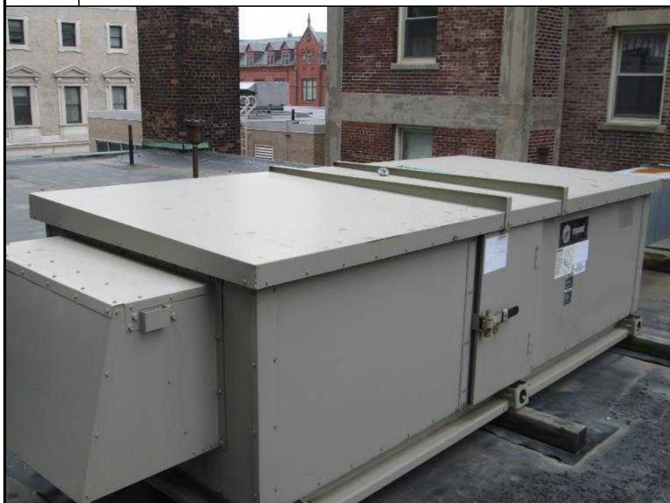
14. Rooftop HVAC unit
