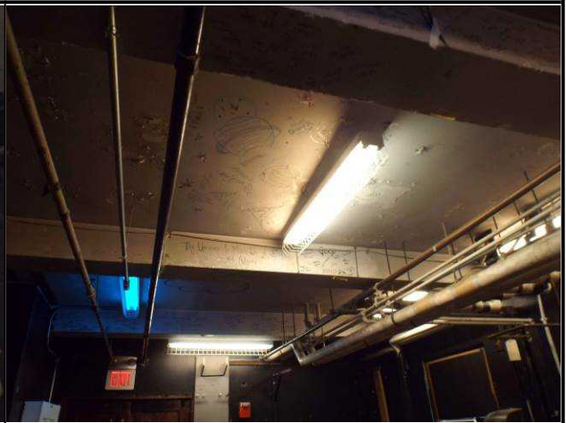
Damaged finishes in "L"
