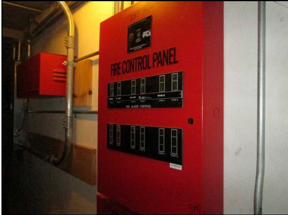
33. 258 Huntington fire control panel
