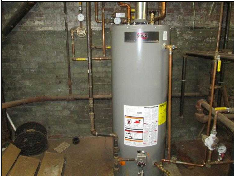
36. 258 Huntington gas water heater
