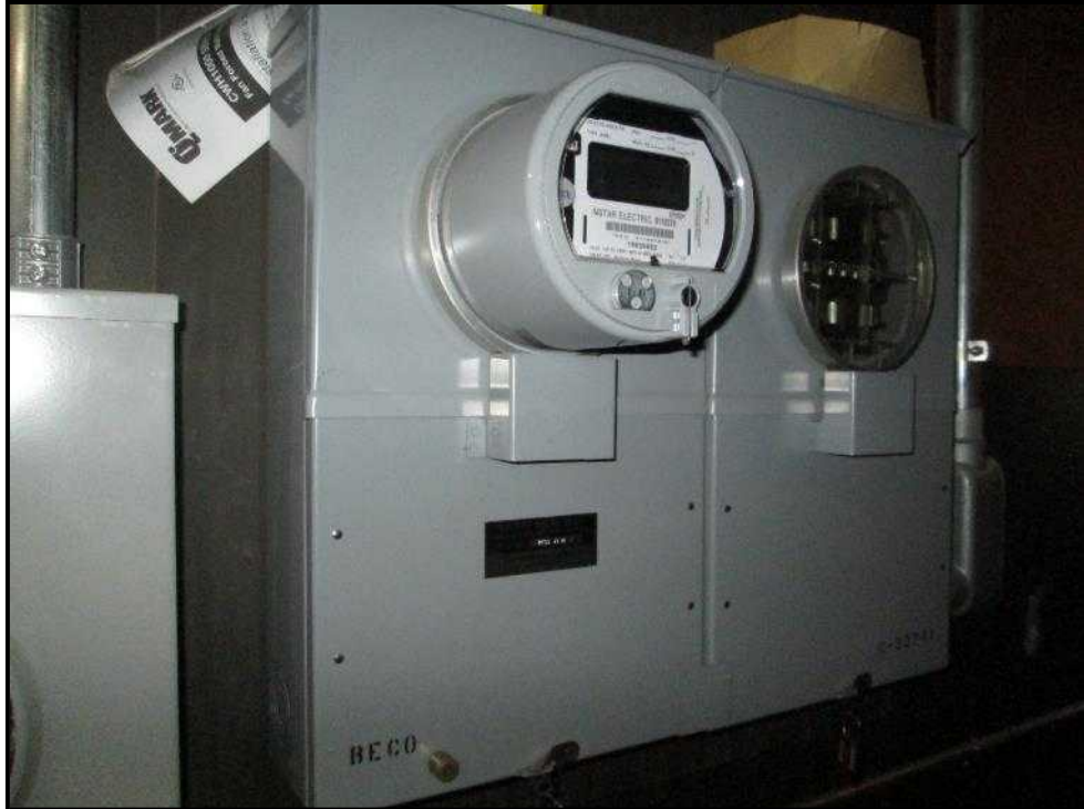
29. Main electrical distribution panel and meter
