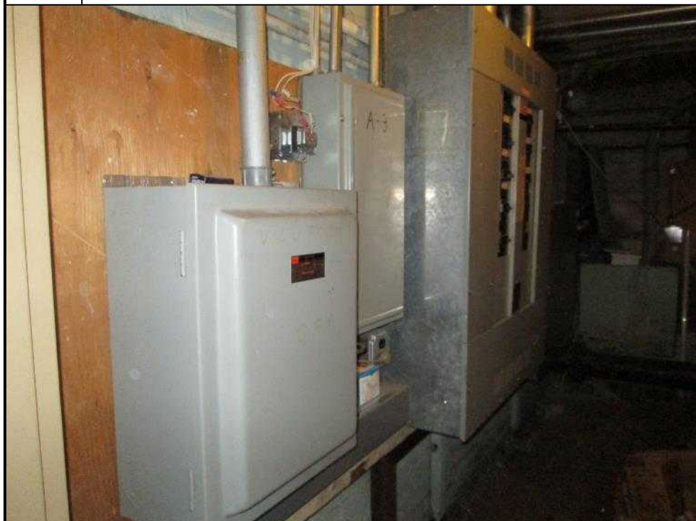
32. 258 Huntington electrical panel
