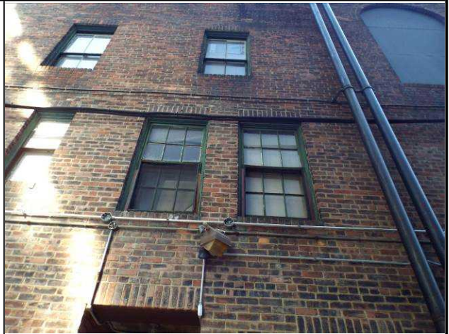
Old, failing windows
