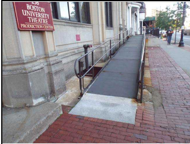
HP ramp with corrosion extending off property
