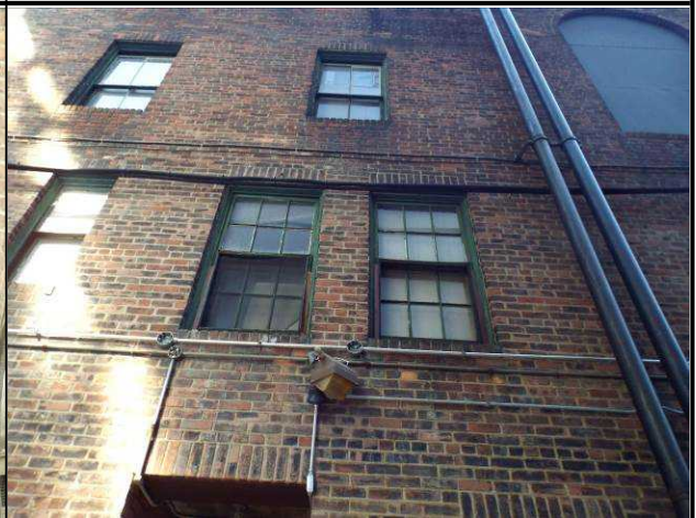
Failed sealants at windows
