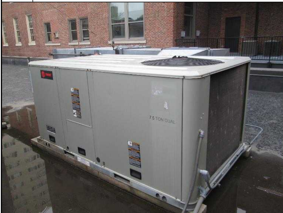
20. 258 Huntington roof top HVAC unit
