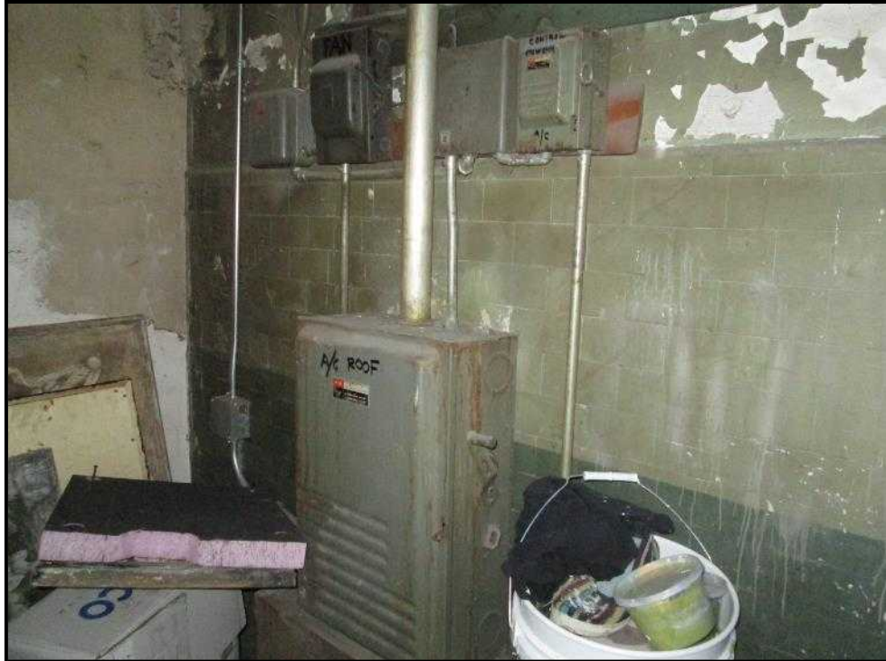
31. 254 Huntington electrical panel
