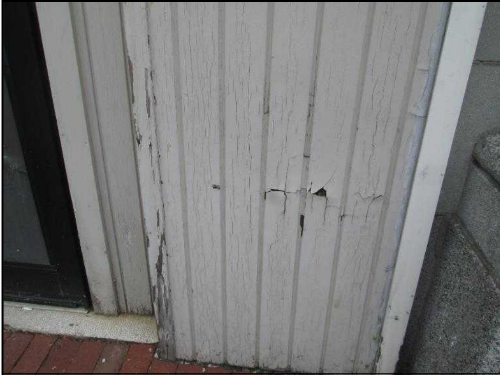
9. Damage wood siding on 252 Huntington
