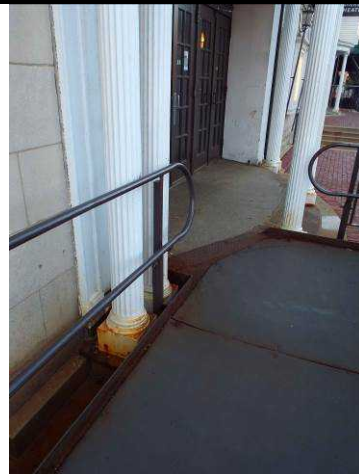
Corrosion at cast iron facade
