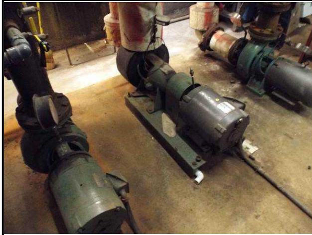
Cooling tower circulation pumps
