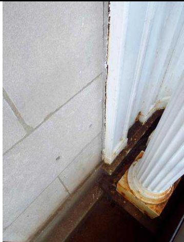
Corrosion and failed sealants
