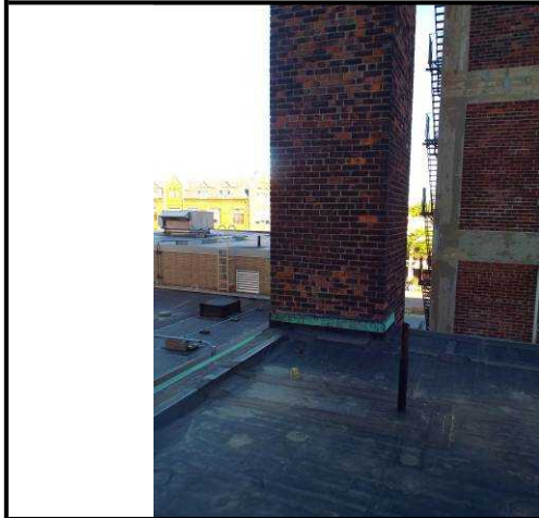
Chimney requiring repointing
