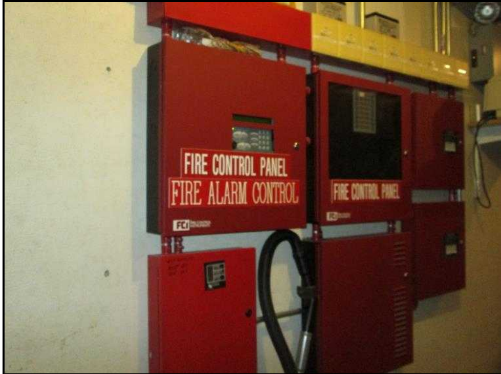
23. Fire alarm control panel
