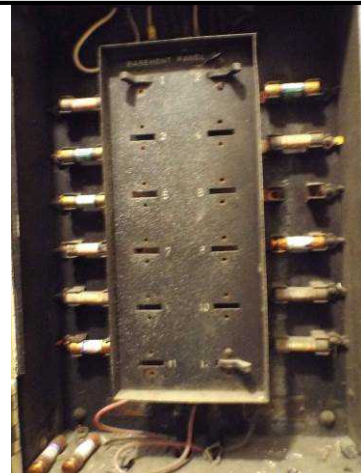
Outdated electrical panel
