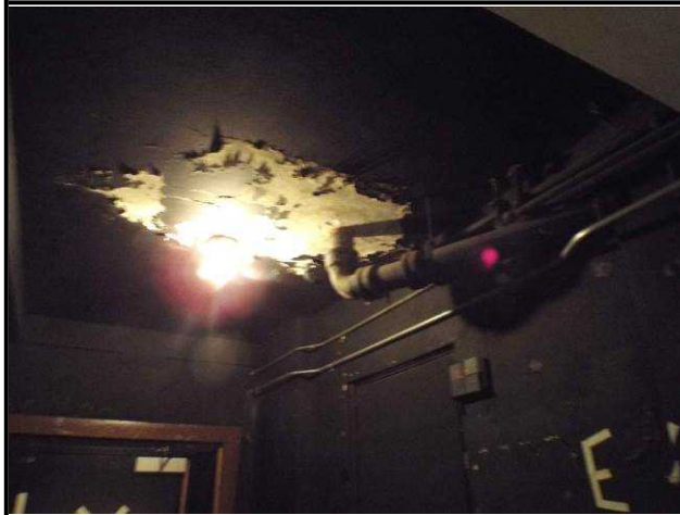
Damaged finishes in "L"
