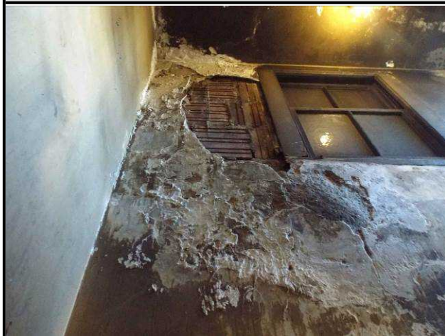
Water damage to stairwell
