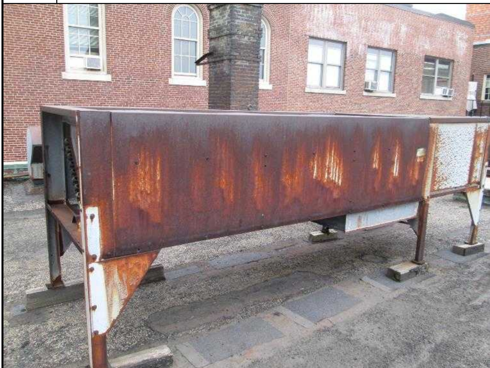
14. 252 Huntington rooftop HVAC unit
