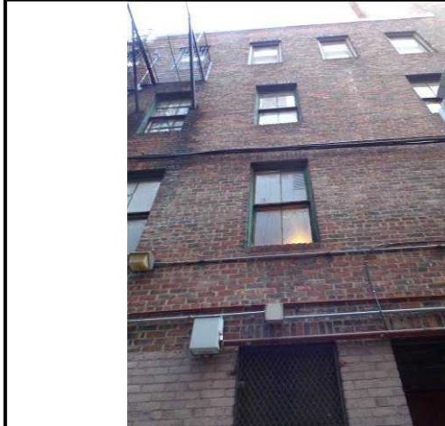
Old, failing windows
