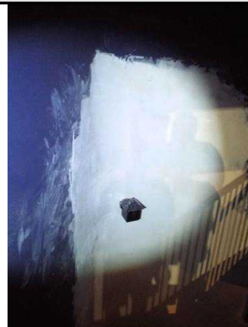
Location of drain pipe failure
