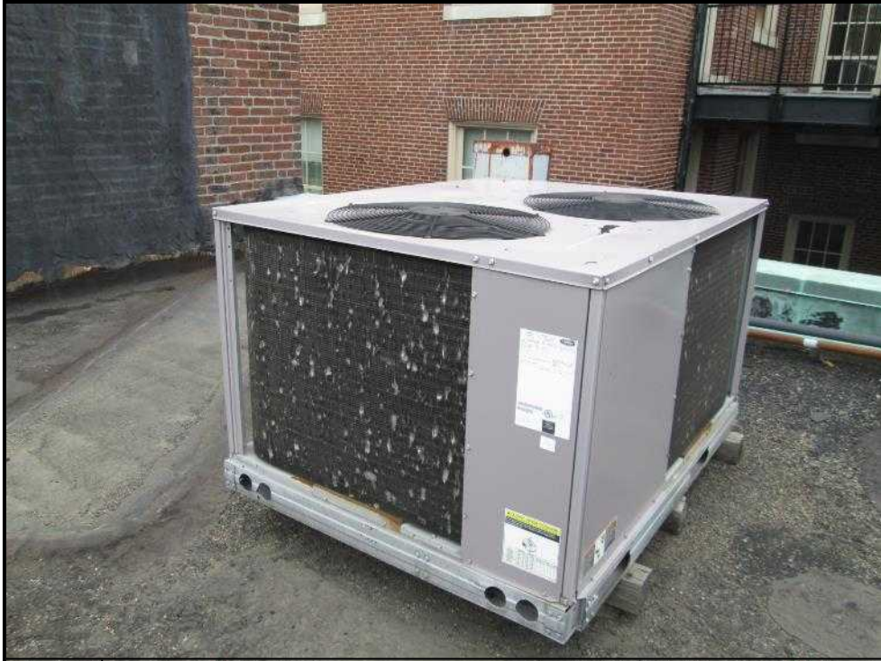
15. 252 Huntington rooftop HVAC unit
