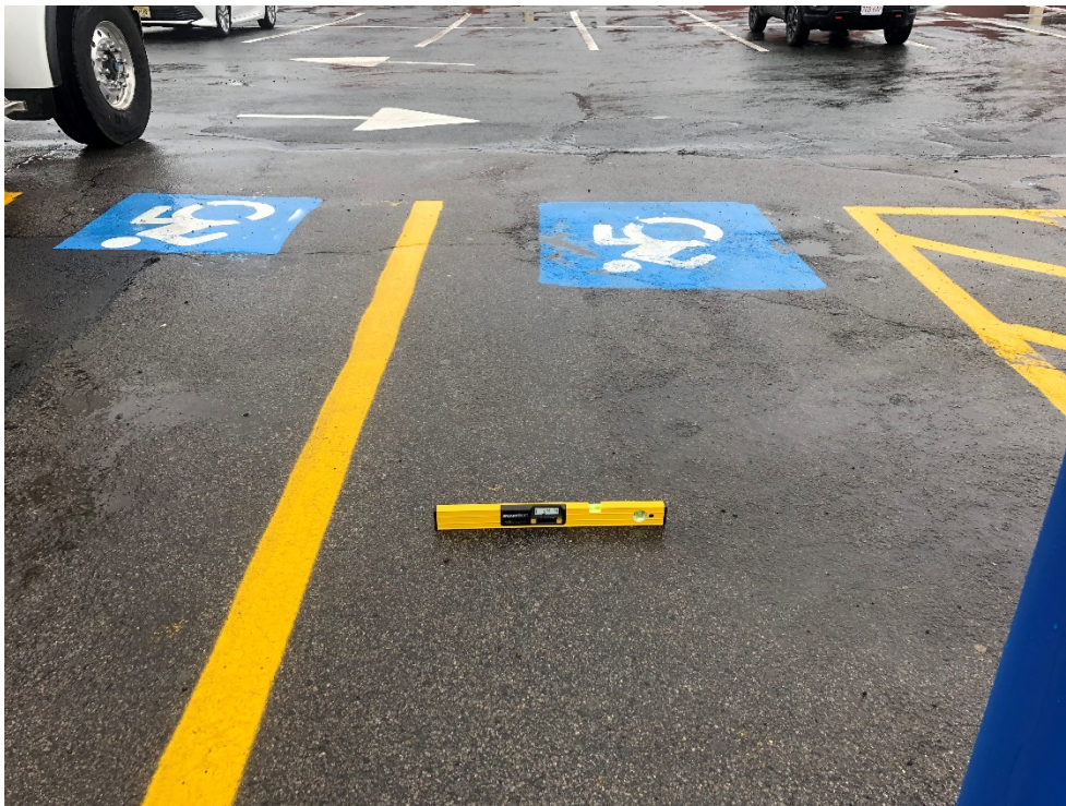
Figure 3.4: Existing ADA Spaces with 3.4% Cross-Slope (2.0% Max. Allowed)
