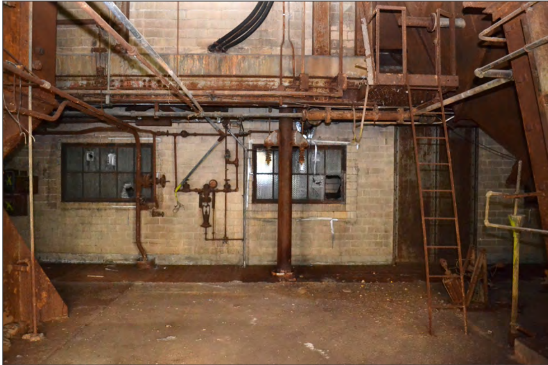
15. Turbine Hall No. 3, facing north
