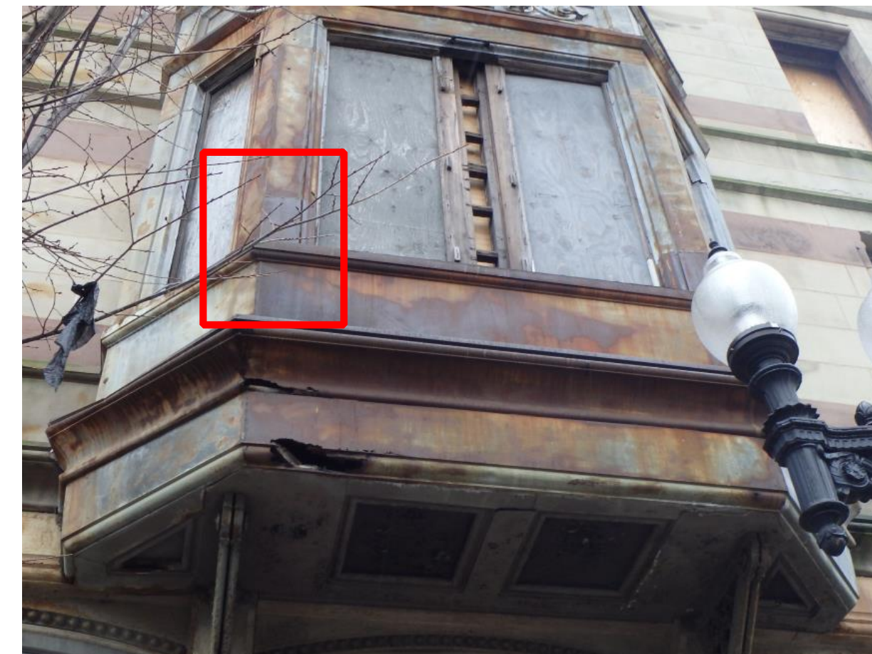
Sheet metal bay Mass Ave north. Note repairs where small balcony was removed.
