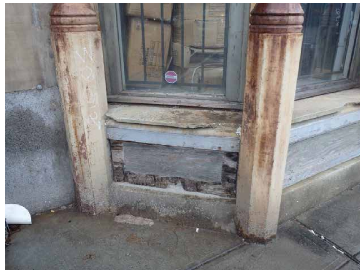
Storefront with replacement cast stone sill and base (date unknown)
