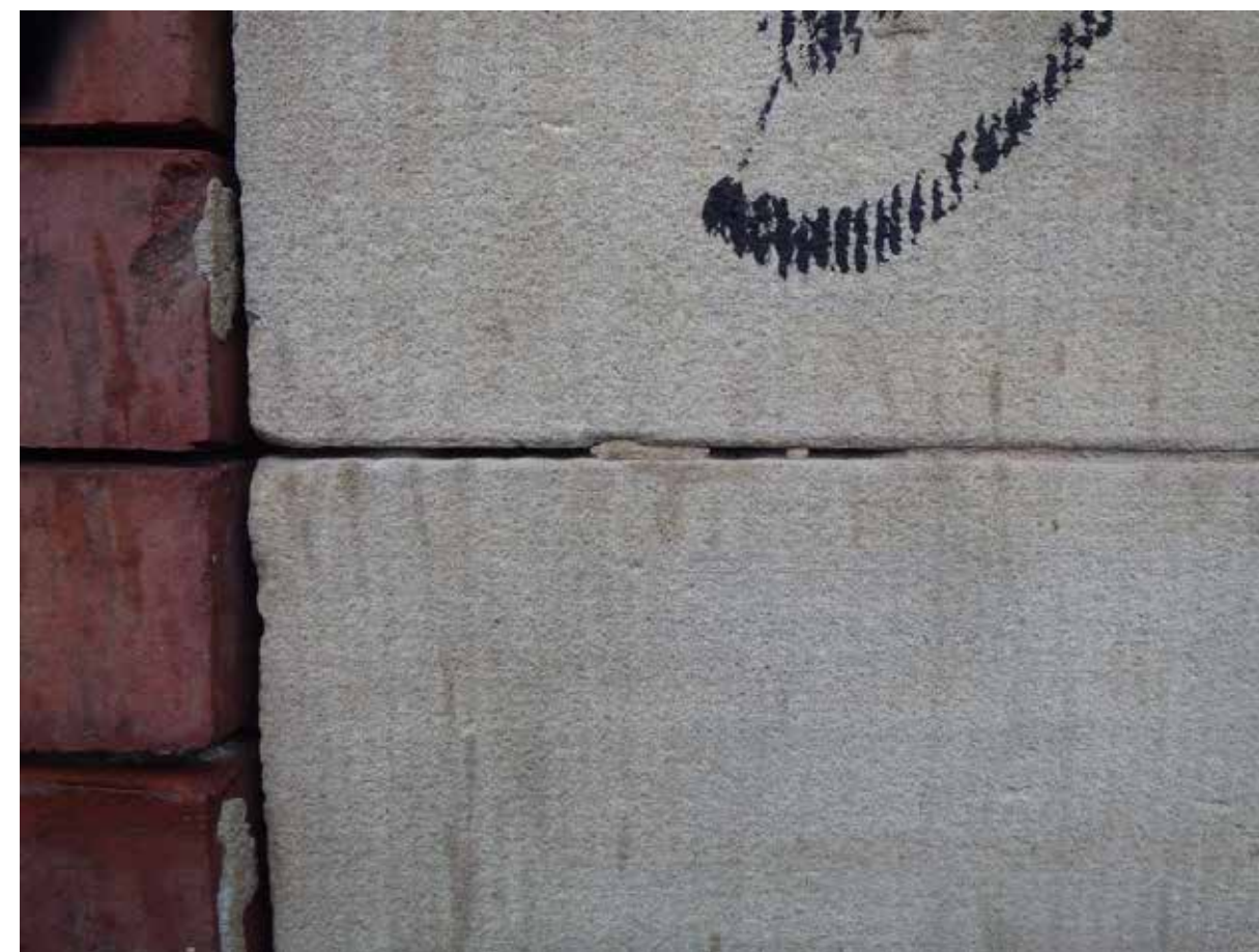
Typical stone joints - narrow and missing mortar
