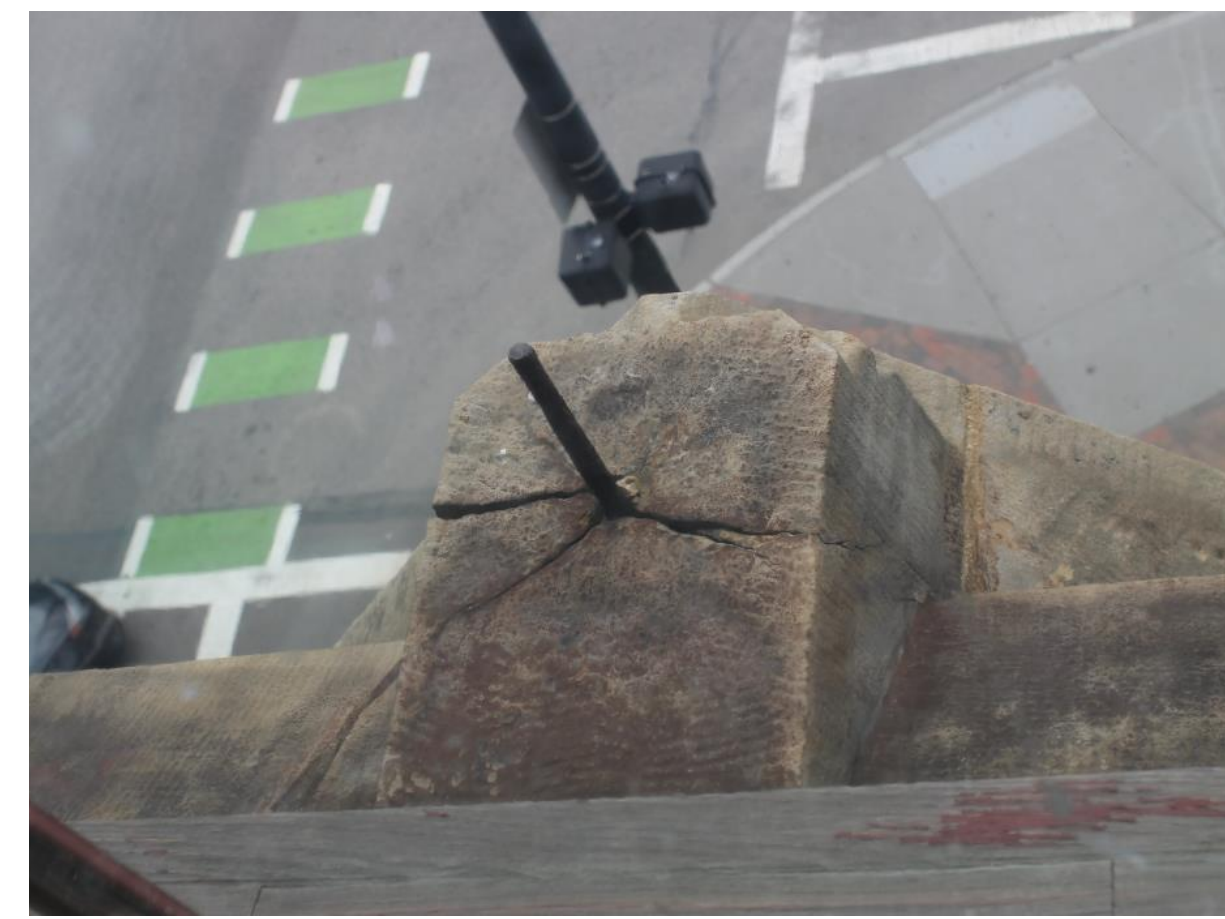
Pin at missing second floor window gable
