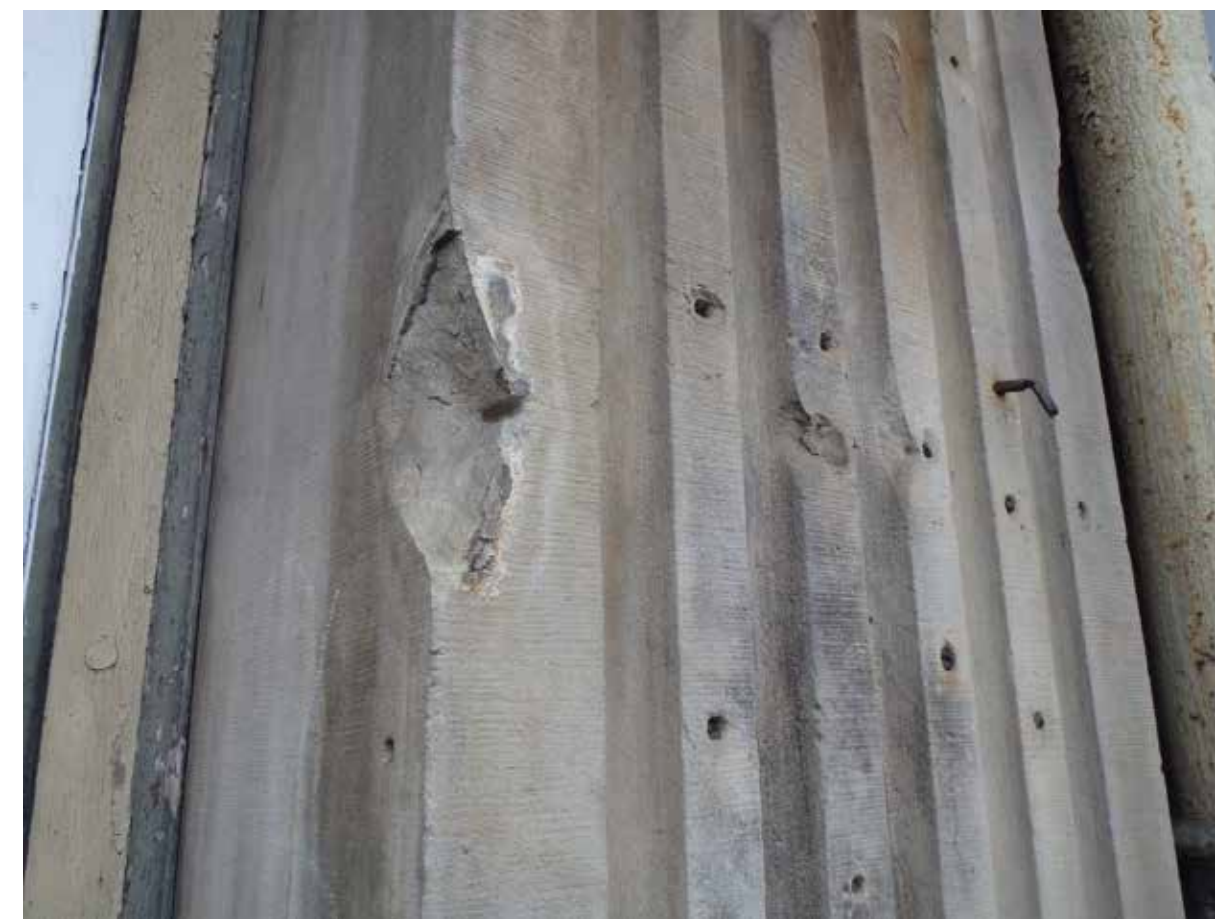
Typical stone damage - spall, anchors, soiling
