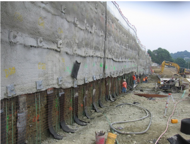
Photo #9. Four lifts of soil nails and shotcrete completed, preparing for fifth lift
