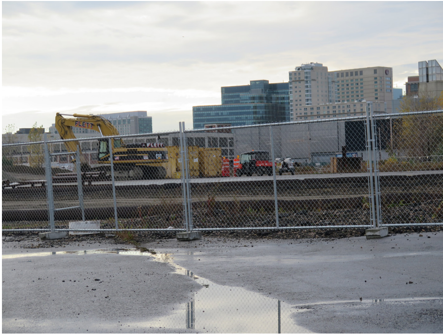
View of Parcel 5 Through Fence on Parcel 6, Showing Tide Street Extension Construction Between Parcels
