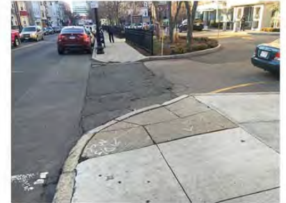
3. Pedestrian ramps at the existing site entrance are not ADA/MAAB compliant. This location will be improved with an at-grade concrete sidewalk crossing with truncated domes to indicate the driveway condition.
