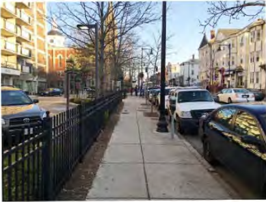
2. The existing City of Boston concrete sidewalk to remain along Tremont Street is in good condition, with ADA compliant slopes and clearances at the tree pits.
