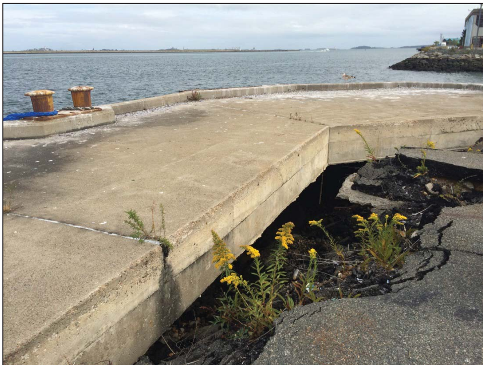
Figure 16: View of open sinkhole in the deck of Dry Dock #4.
