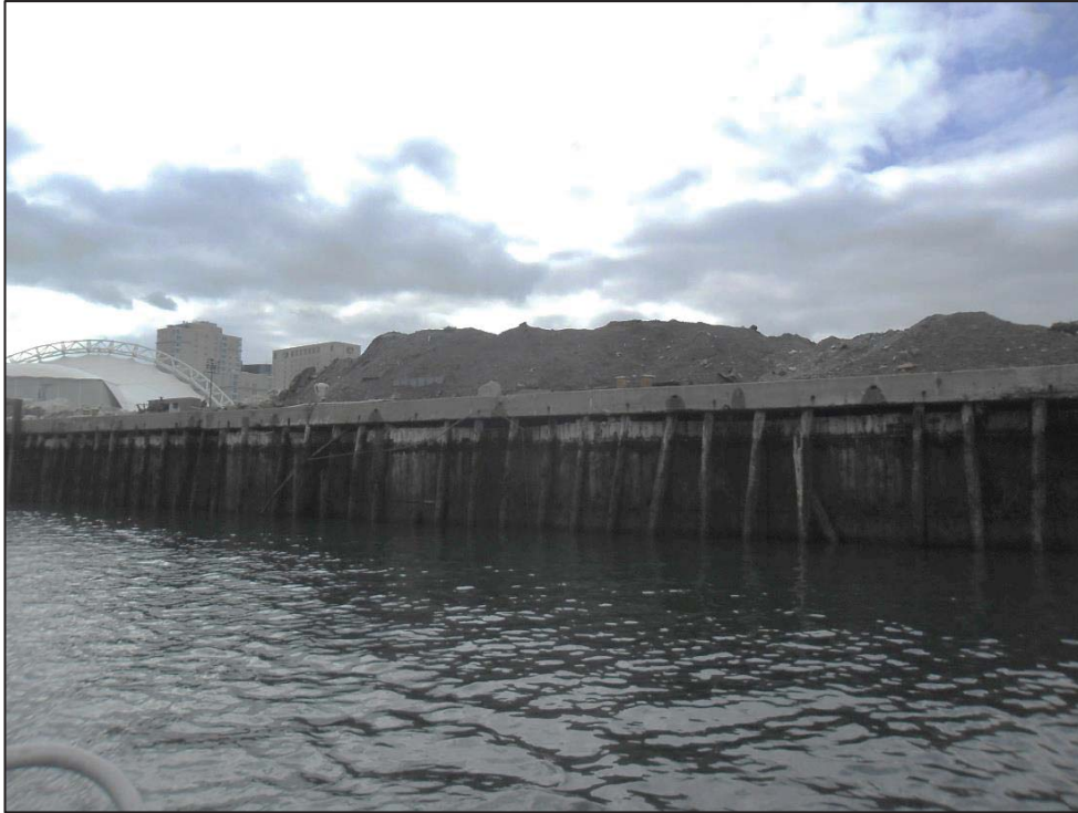
Figure 19: View of the east side of Dry Dock #4. This facility was used for the City's excess snow storage during the harsh winter of 2015.
