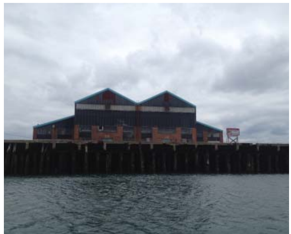
Parcel M remains unoccupied and in need of waterside infrastructure repairs.
