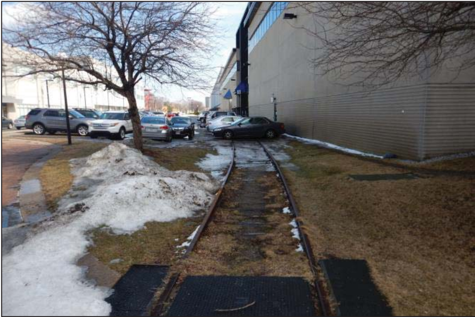
Figure 4: View of existing Track 61 rail which runs adjacent to the Design Center Buildings.
