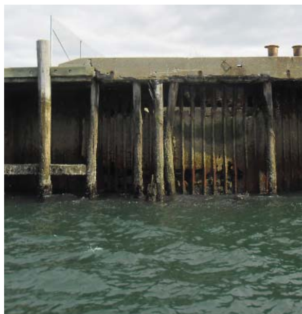
Damage to the South and East Jetties has reduced their structural capacity.
