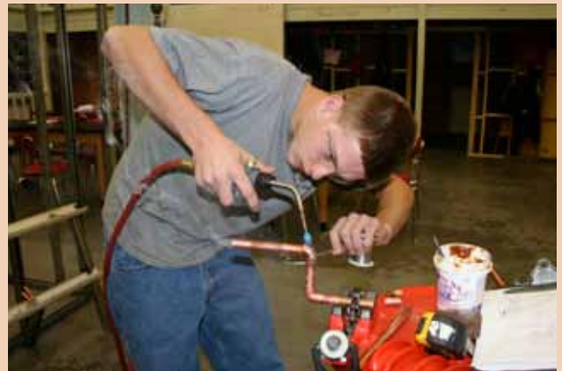
A student receives training in plumbing, one of the vocational programs in construction trades at Shawsheen Valley Technical High School in Billerica, MA. The school, which opened in 1970, has a population of more than 1,300 students.
