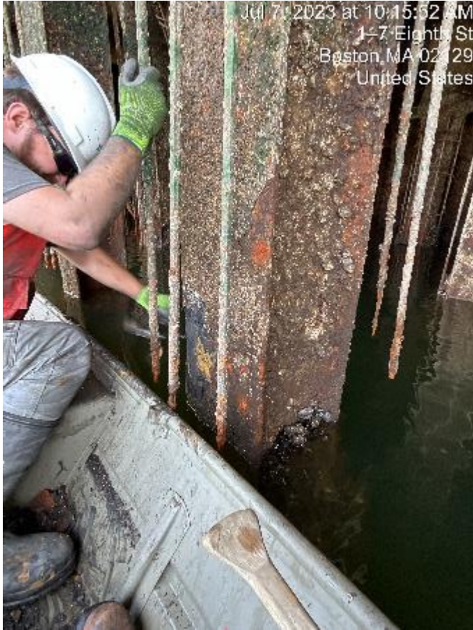
Minor Damage 0%-15% Steel Loss 30% of Piles
