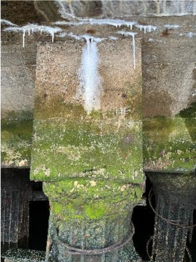
Minor Damage 8% of Caps Small Cracks
