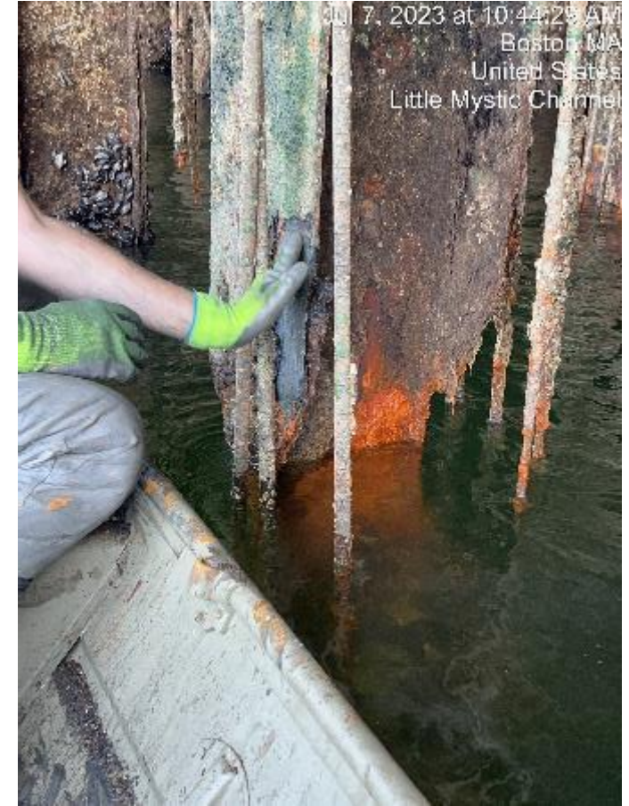
Severe Damage 50%-100% Steel Loss 36% of Piles
