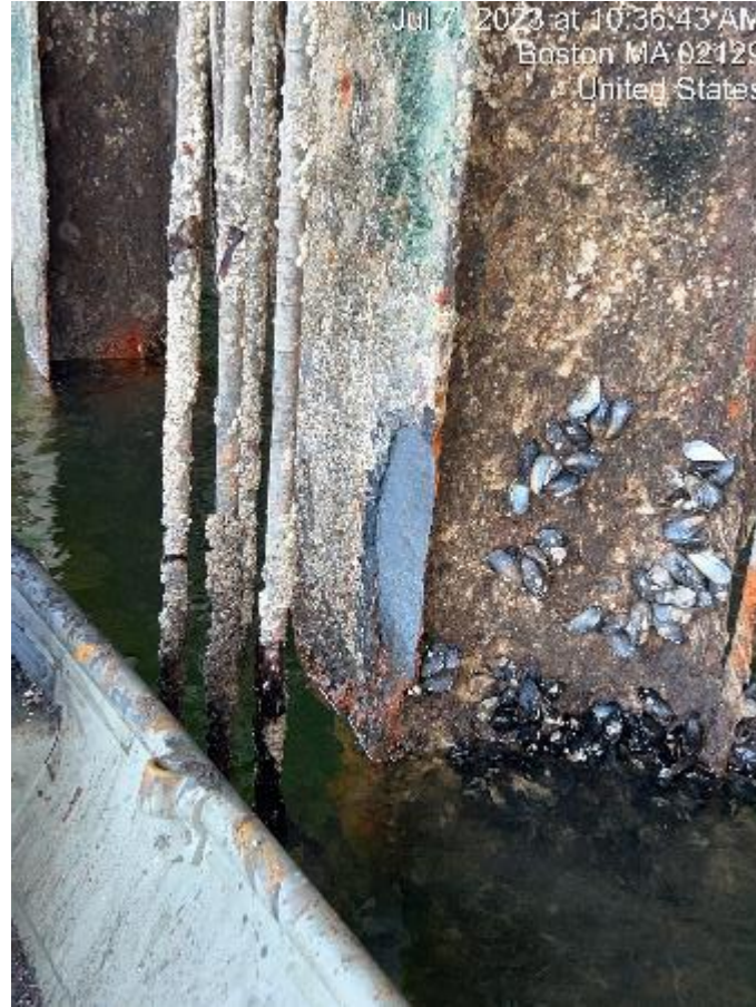
Major Damage 30-50% Steel Loss 21% of Piles
