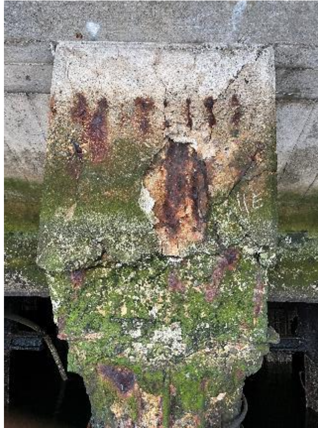
Major Damage 74% of Caps Exposed Reinforcement
