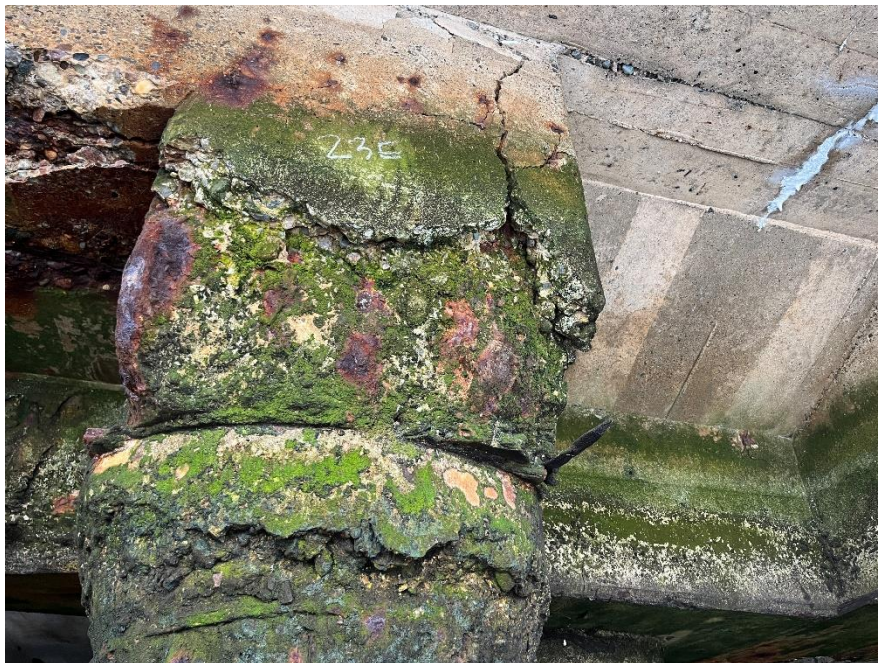
Figure 4 Example of "Severe" damage pile cap. Corresponds to corrected pile 30E on the Foth pile plan. Note exposed reinforcement due to chemical deterioration and structural cracks >1/4 ".
