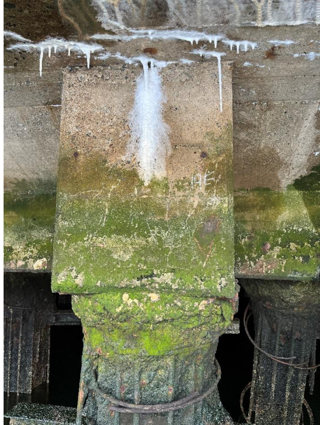
Figure 5 Example of "Minor" damage pile cap. Corresponds to corrected pile 26E on the Foth pile plan. No visible corrosion cracks or chemical deterioration. Note corrosion stains and non-structural cracks <math>< 1/16</math>".
