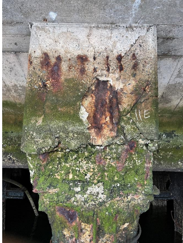
Figure 3 Example of "Major" damage pile cap. Corresponds to corrected pile 18E on the Foth pile plan. Note exposed reinforcement and chemical deterioration with structural cracks.
