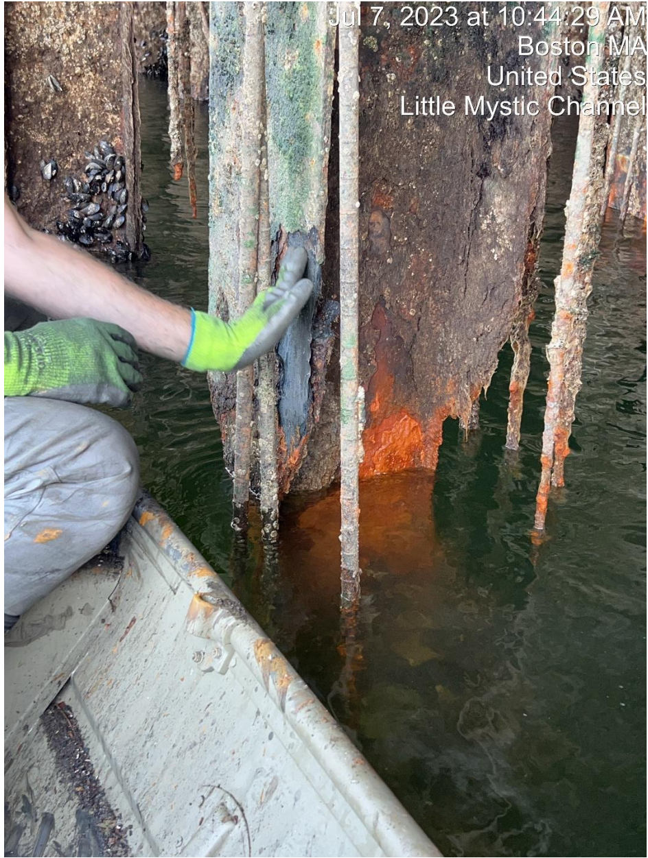
Figure 10 Pile 102-W, another example of a Severe damage pile. 0.13" of steel measured, 82% loss. Complete loss of flange just below waterline.
