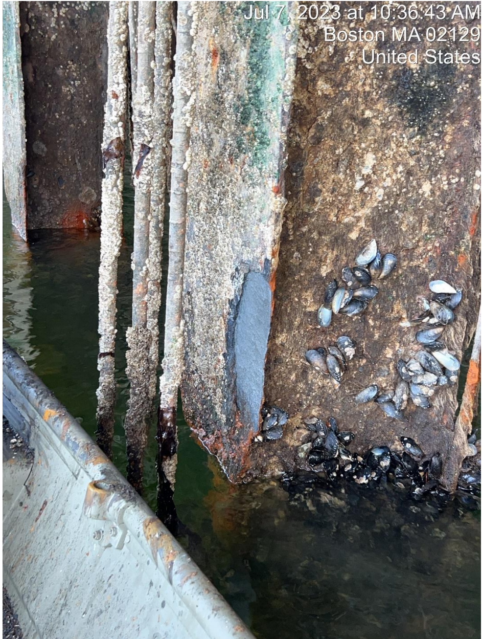
Figure 8 Pile 111-W, and example of a Major damage pile. Measured steel thickness of 0.47", 33% loss. Note the knifed edge that has corroded almost all the way through.
