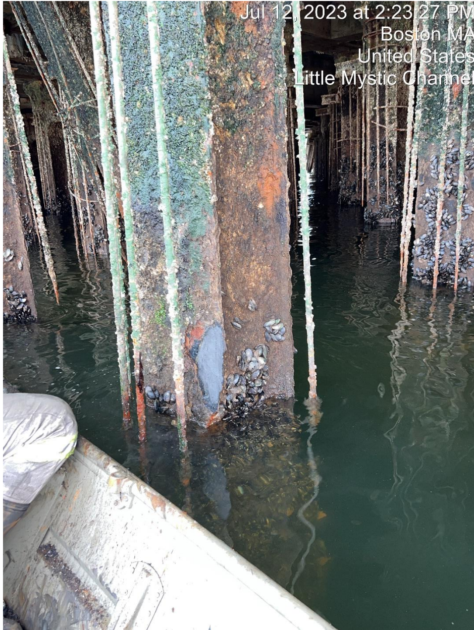
Figure 9 Pile 103-E, example of a Severe damage pile. Measured thickness of .015", 79% loss. Below the waterline it was noted that corrosion goes all the way through the flange.
