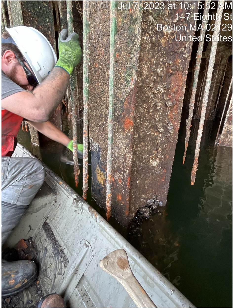
Figure 6 Minor damage H-pile example, pile 38-W on the Foth plan.
