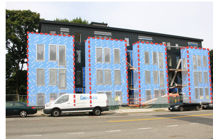
Article 80 project under construction at 59-63 Belgrade Avenue, which includes 3-story bays to minimize scale
