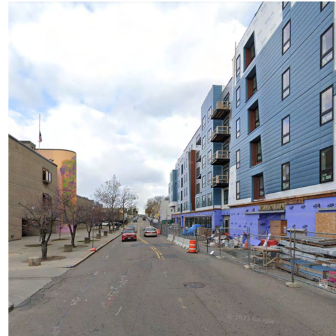
FIG 03-26 BORDER STREET LOOKING NORTH. (2022) [BOTTOM LEFT] At right, construction of 301-303 Border Street, a mixed-use mid-rise project that includes 64 dwelling units and ground floor commercial space. At left, the Mario Umana Academy, a Boston Public School.
