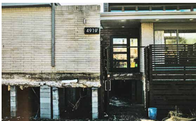
Construction photo showing house elevating on extended foundations. Spaces below SLR-DFE are not habitable.
